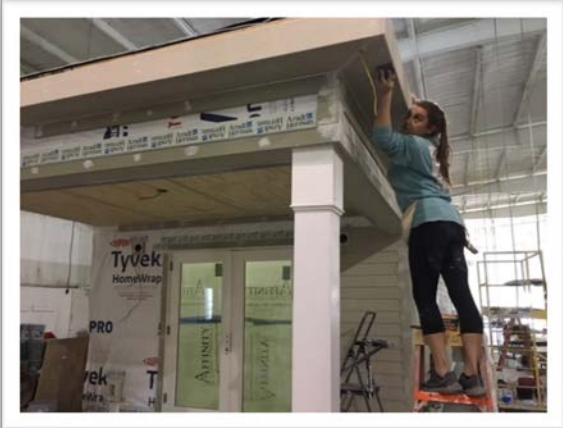
Below left, a modular plant worker constructs the porch soffit during a plant visit by CHSA and City officials.
