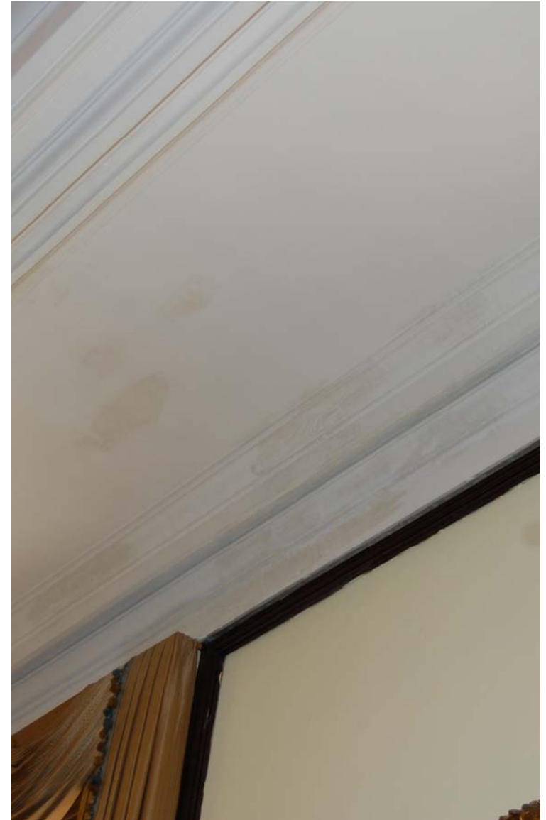
Water damage located on south ceiling. Figure 64
