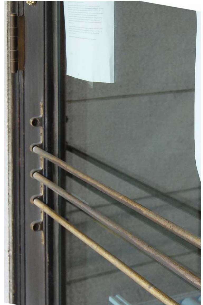
Front entrance door showing missing brass hardware.
