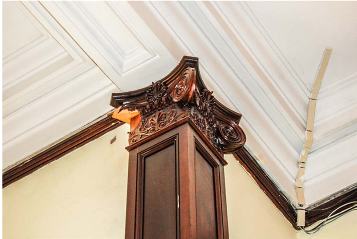
Missing ionic scroll from engaged column capital in Council Chambers at southwest corner.
