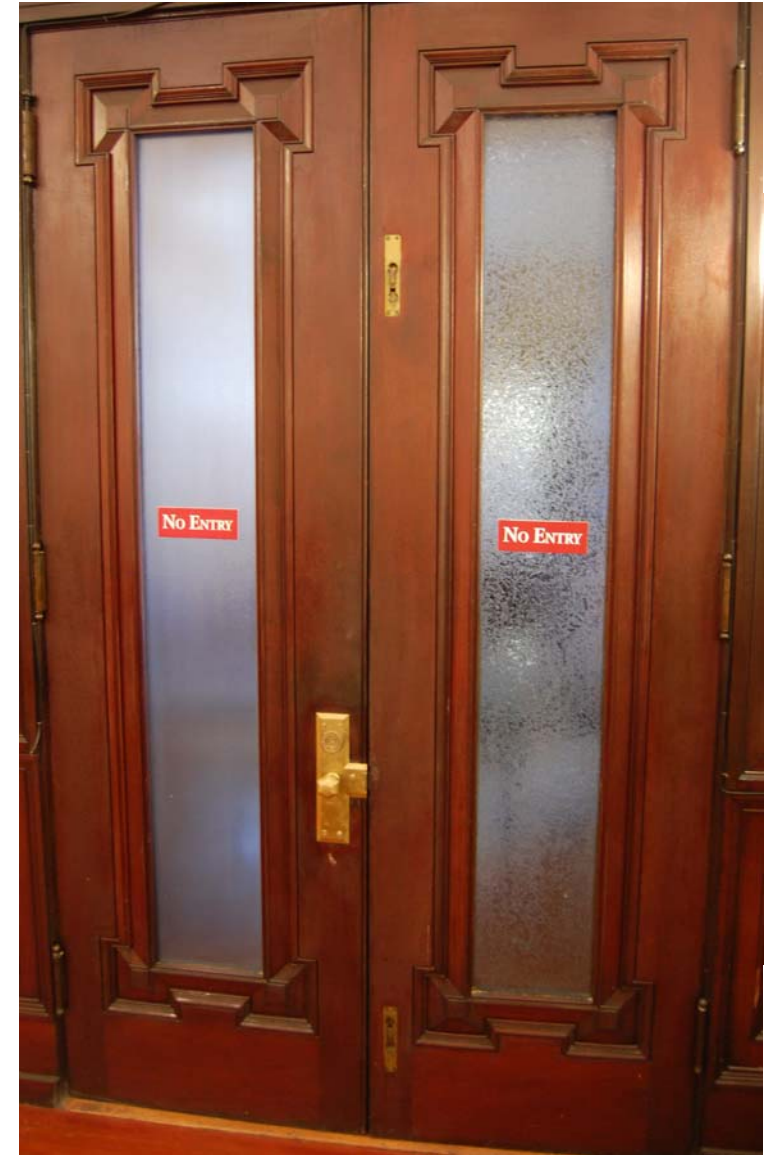
Doors leading from Council Chambers to the Reception Room, each of which has a different type of etched glass. Figure 84
