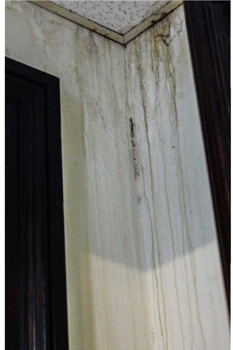
Detail of water damage in Rotunda alcove corner. Figure 48
