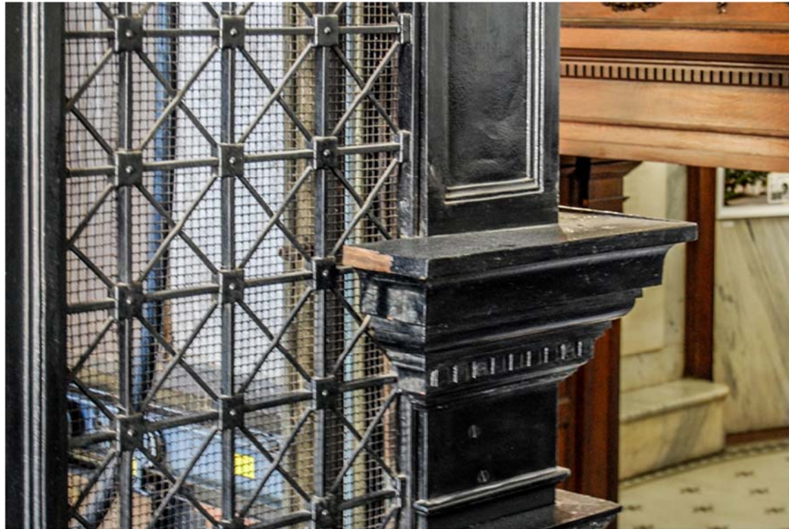
Location of missing paint on elevator column capital detail. Figure 15
