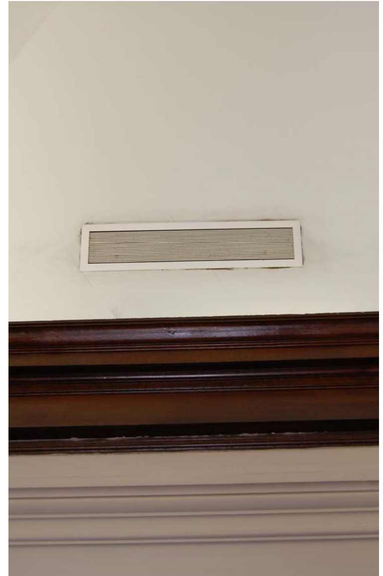
Abandoned air intake vent in Reception Room ceiling. Figure 83
