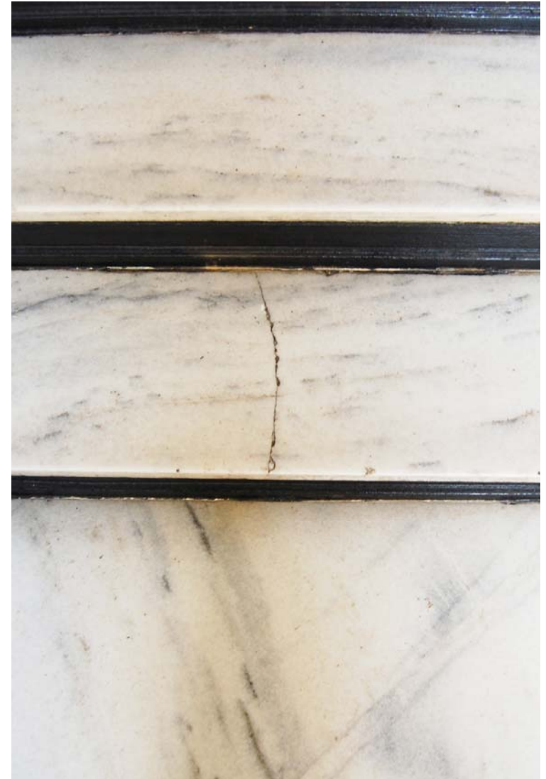
Detail of cracked marble stair tread. Figure 60
