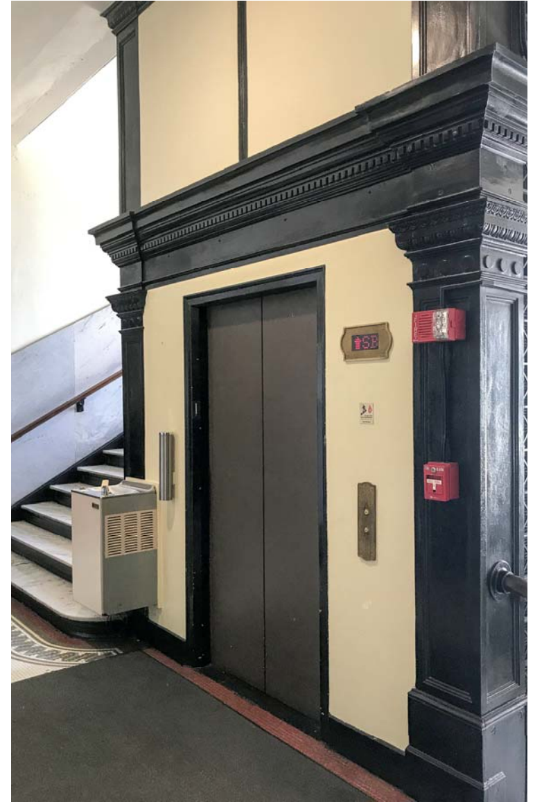
Detail of elevator entrance on the first floor in its current configuration. Figure 56
