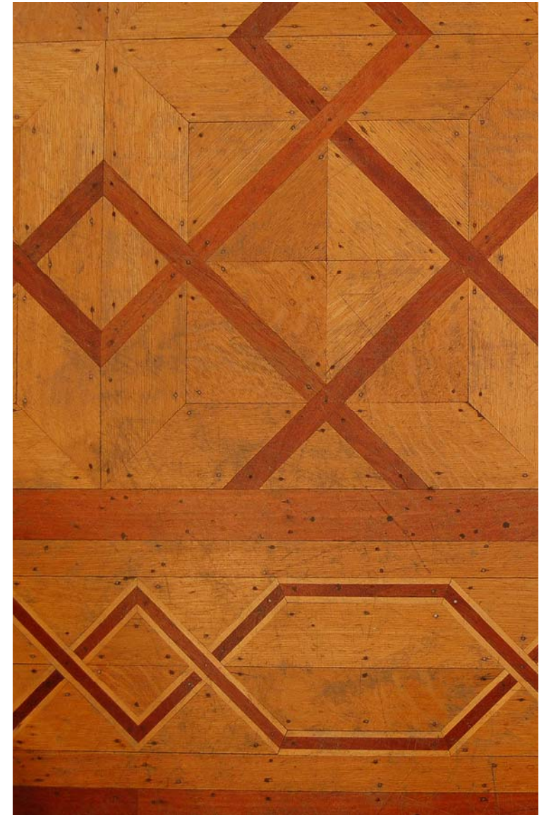
Parquet flooring in Council Chambers showing scratches and scrapes. Figure 68
