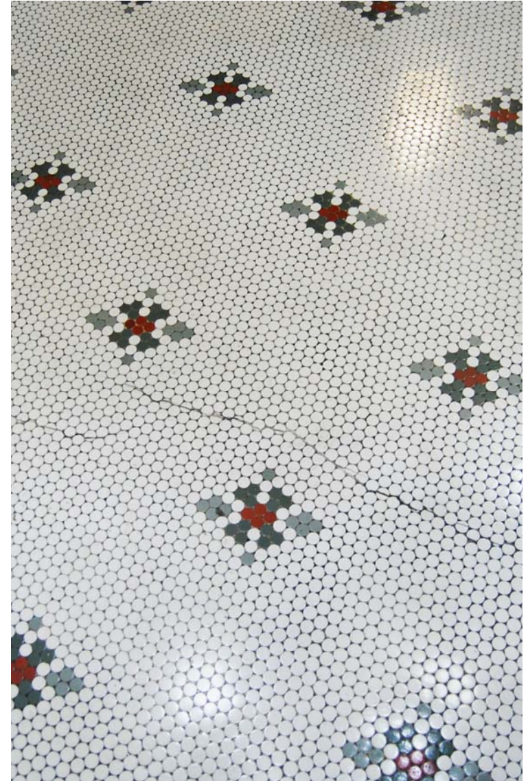
Floor cracks at the first floor level of the Rotunda. Figure 45
