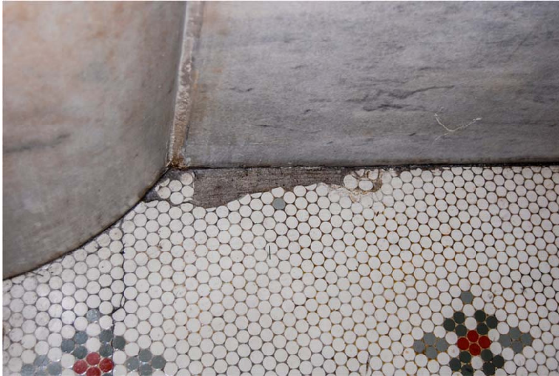
Tile loss in northeast alcove on east wall of first floor Rotunda Figure 7
