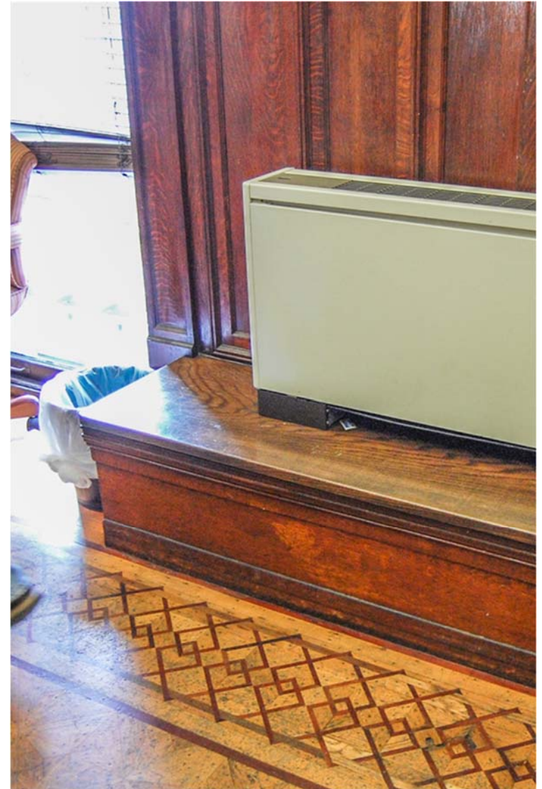
Modern HVAC units mounted to historic benches on south wall of Reception Room. Figure 25
