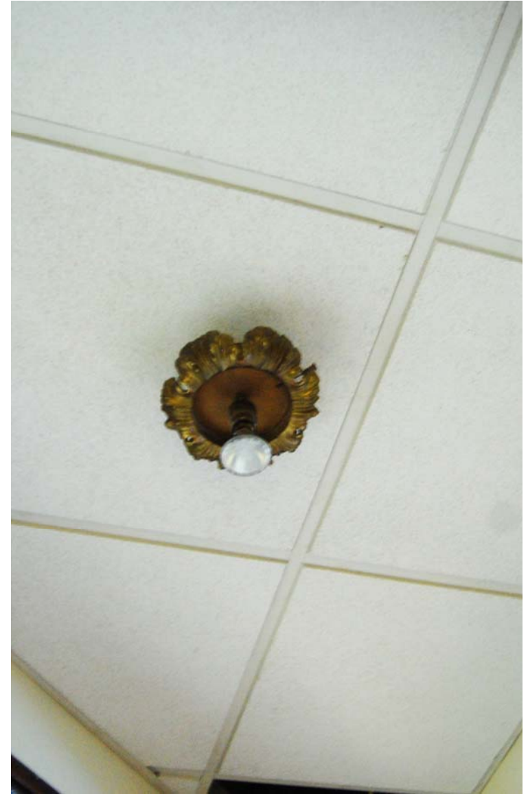
Original light fixture missing its globe, surrounded by replacement drop ceiling tiles in Rotunda alcove. Figure 50
