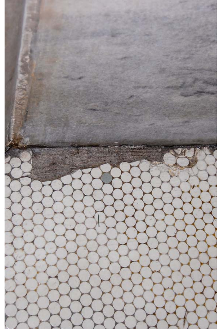
Missing penny tile in northeast alcove of Rotunda. Figure 44
