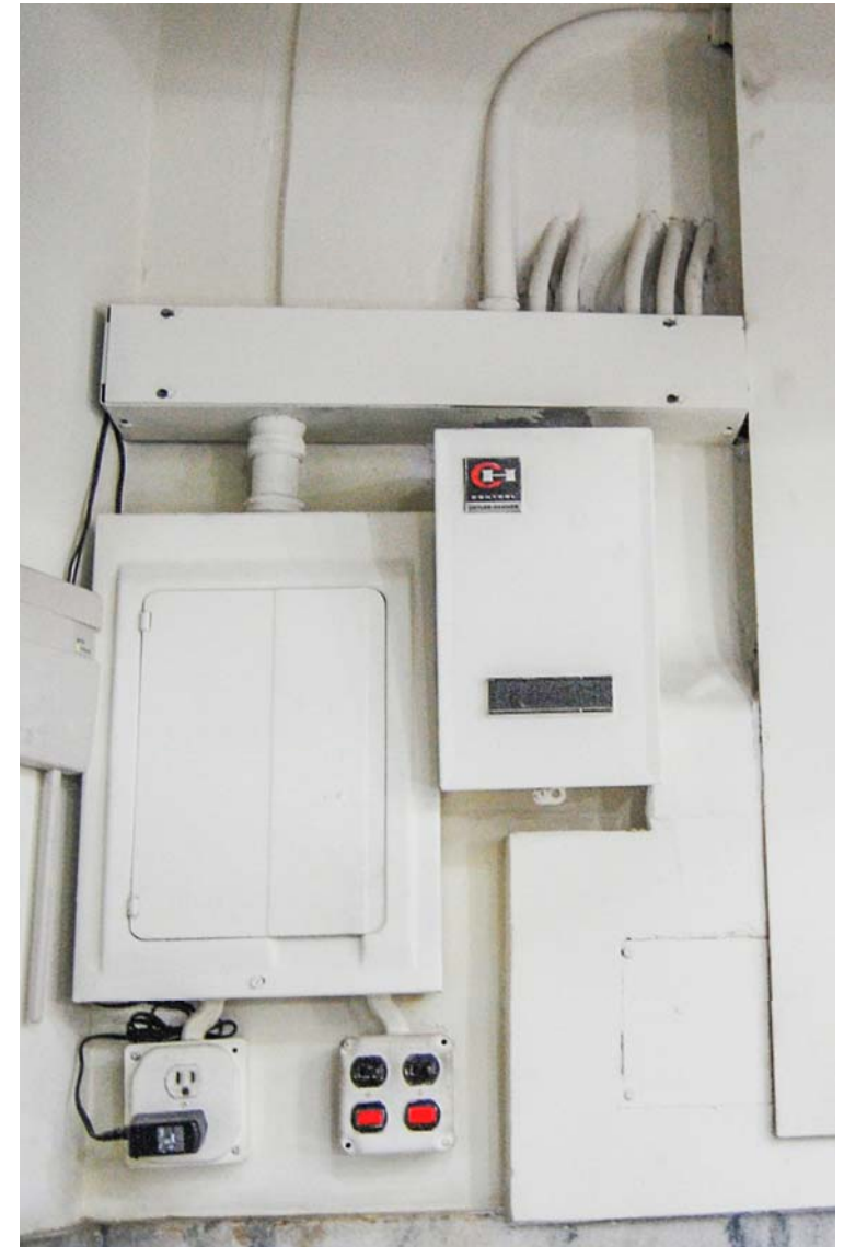
Some of the many electrical panels in the southwest alcove of the Rotunda. Figure 51
