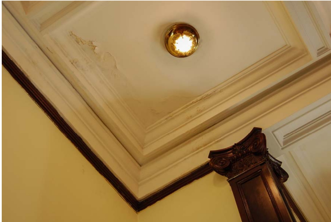
Detail of ceiling coffer plaster damage at southeast corner of Council Chambers. Figure 21
