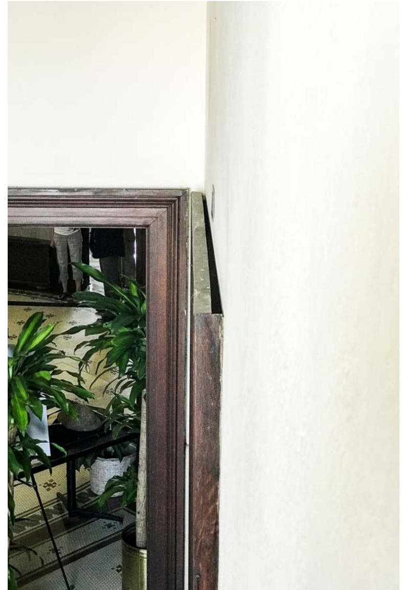
Detail of unsecured framing of entrance into the Municipal Records and Archives off the first floor Corridor on west wall. Figure 13
