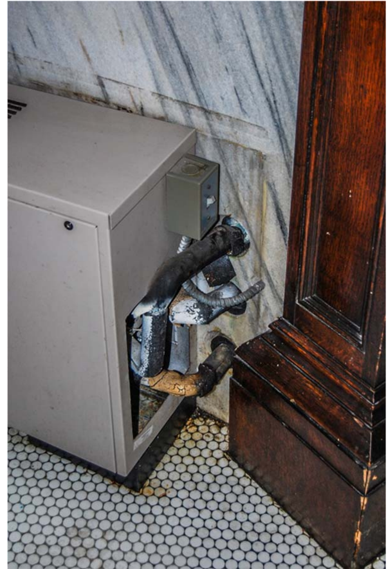
Detail of HVAC connection on South wall in Second Floor Rotunda. Figure 10
