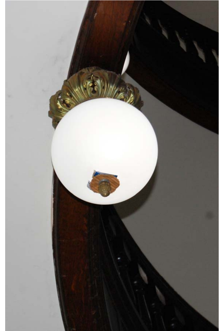
Original brass globe light fixture that has been altered. Figure 49
