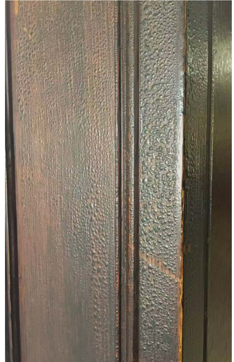
Detail of stain on wood door frame in Rotunda. Figure 43
