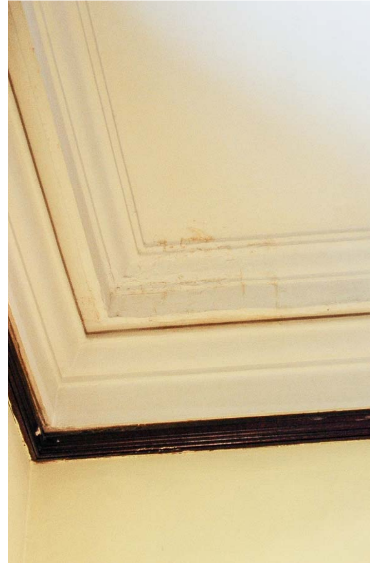
Water damage located on south ceiling. Figure 65
