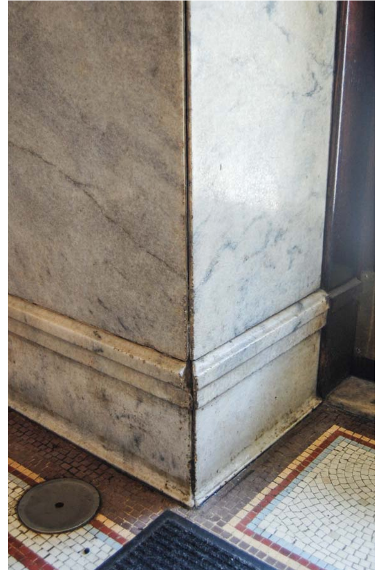
Marble separation at corner of wall panels in Lobby.
