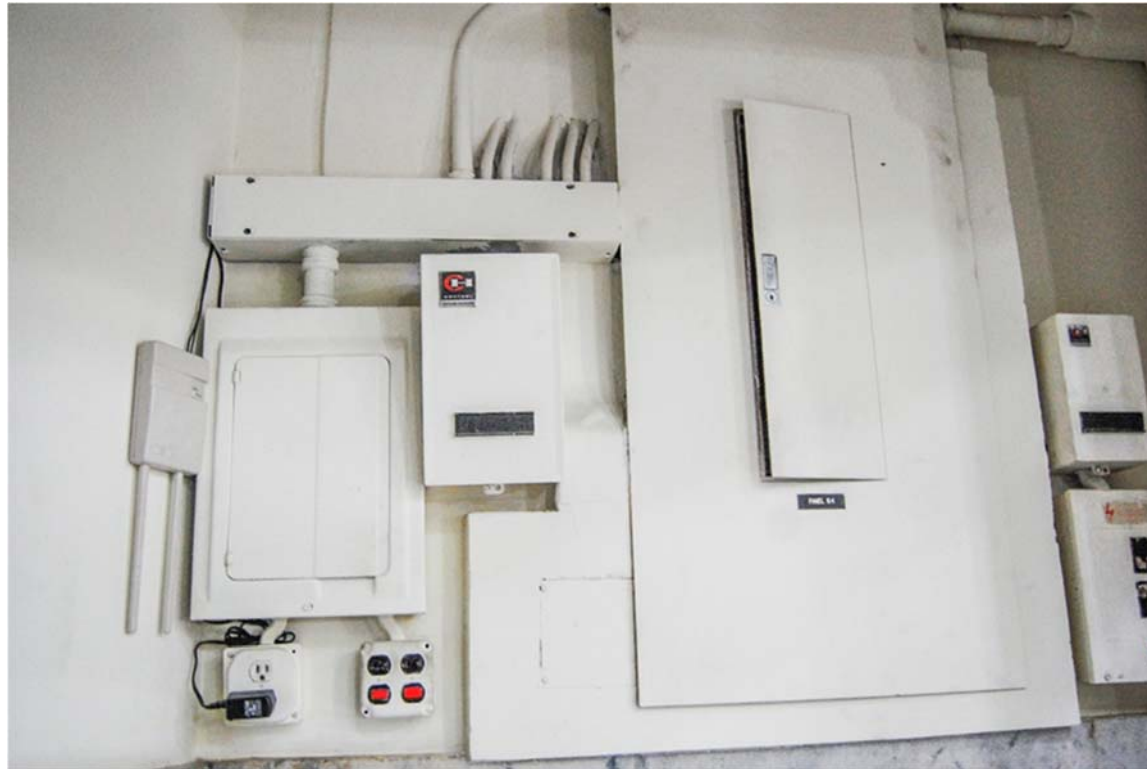
Electrical panels on west wall of southwest alcove in second floor of the Rotunda.
