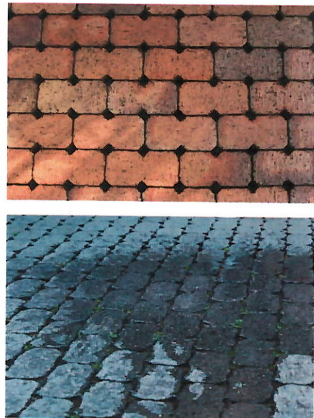
Figure 5.14. Examples of permeable pavers.
