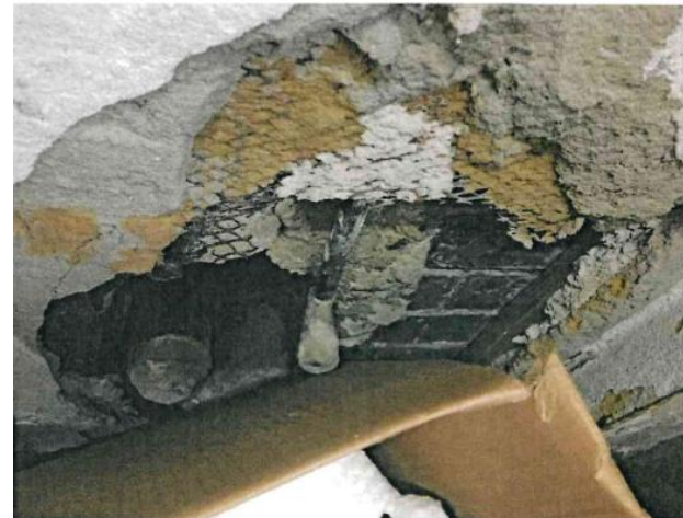
Plaster deterioration and openings in wall
