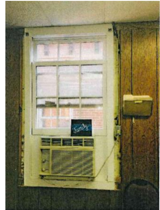
Window units causing moisture accumulation and mildew
