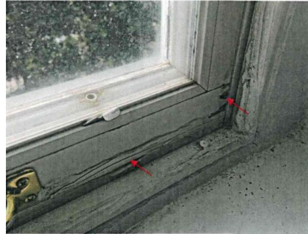
Window moisture damage containing rot
