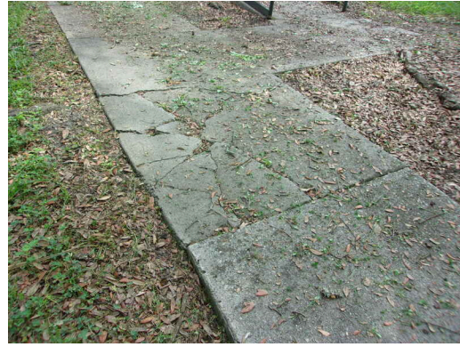
Typical damaged concrete sidewalk with trip hazards (Critical Repair)
