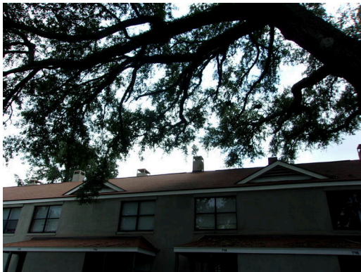
Typical trees touching apartment building roofs (Non-Critical Repair)
