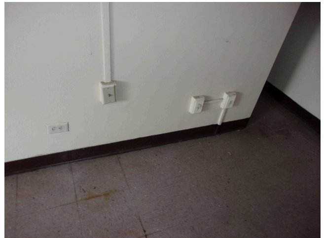
4. 121-128 Yamacraw Village - Unit 126 - 2-bed/ 1-bath TH - Cable and electrical outlets
