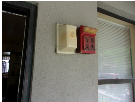
260-268 Yamacraw Village - Unit 261 - 1-bed/ 1-bath - HC unit - Emergency call light and fire alarm
