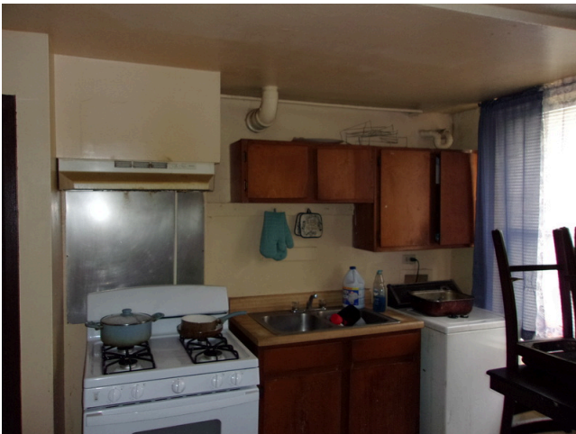
19. 141-148 Yamacraw Village - Unit 142 - 3-bed/ 1-bath TH - Kitchen view, replace old cabinetry (Non-Critical Repair)
