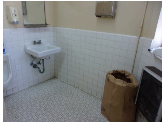
349 West Bryan Street - Community center - Men's restroom - Install scald and abrasion protection (Critical Repair)
