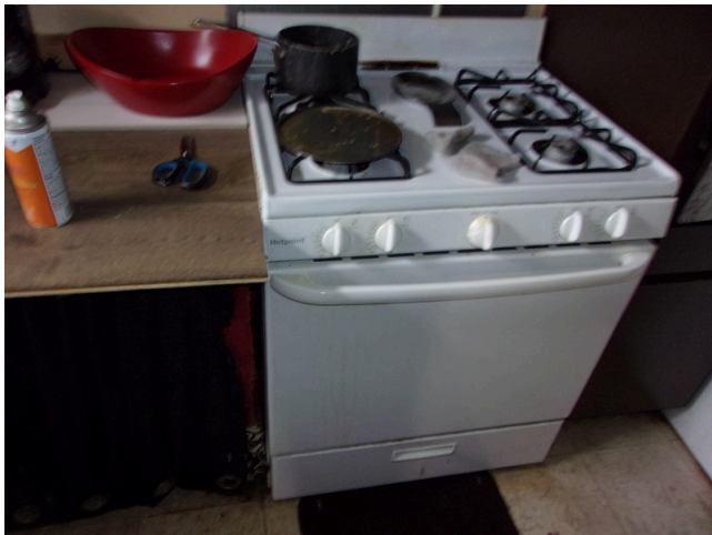
39. 260-268 Yamacraw Village - Unit 261 - 1-bed/ 1-bath - HC unit - Front control range/oven
