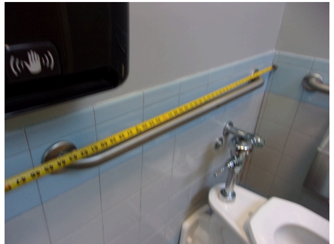
128. 349 West Bryan Street - 2nd floor Doctor's office - Women's public restroom - Compliant rear grab bar
