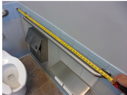
349 West Bryan Street - 2nd floor Doctor's office - Women's public restroom - Compliant side grab bar
