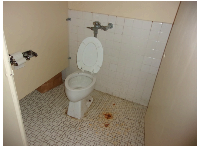
140. 349 West Bryan Street - Community center - Women's restroom - Replace common restroom accessories (Non-Critical Repair)
