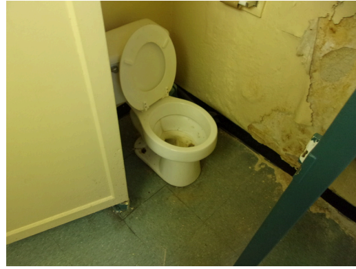
349 West Bryan Street - Community center - Water-damaged interior walls (Non-Critical Repair)
