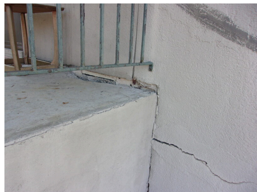
Front porch sinking (Non-Critical Repair)
