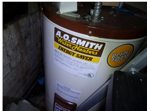
555 West Bay Street Office - Replace old 20-gallon water heater (Non-Critical Repair)
