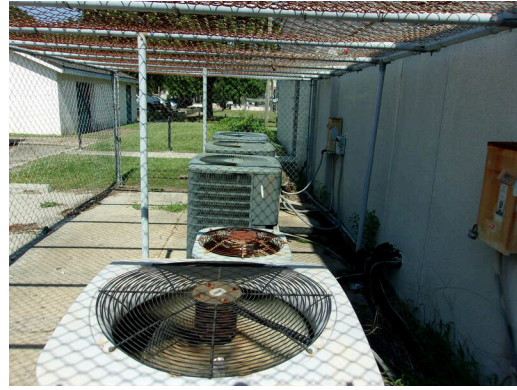
Heat pump condenser units
