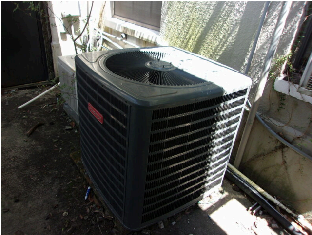
161. 349 West Bryan Street - Heat pump unit
