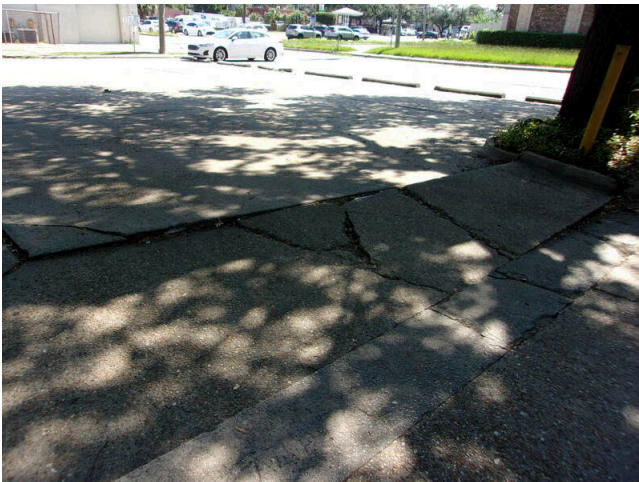
15. Replace heaving and cracked concrete parking lot (Non-Critical Repair)
