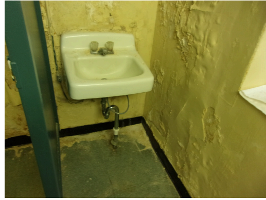
349 West Bryan Street - Community center - Staff restroom with no scald and abrasion at the sink (Critical Repair)
