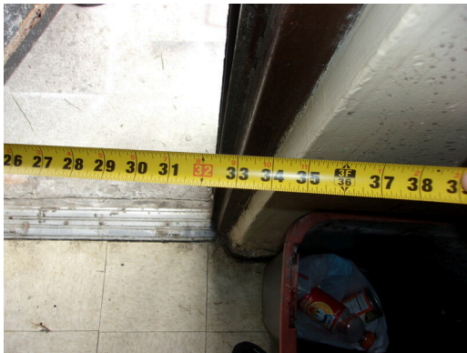
260-268 Yamacraw Village - Unit 261 - 1-bed/ 1-bath - HC unit - 32 inch clear opening at rear door
