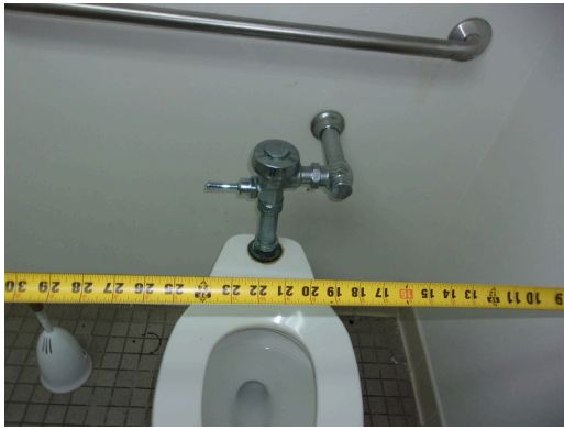
555 West Bay Street Office - Men's public restroom - Clear floor space at toilet
