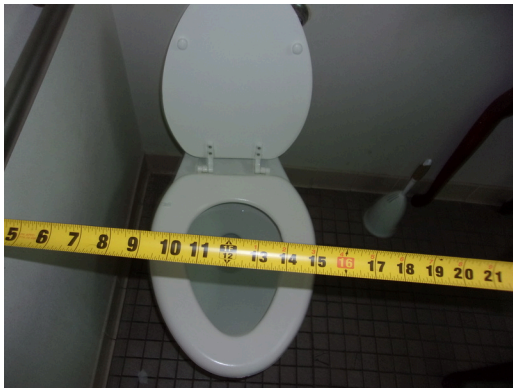
555 West Bay Street Office - Women's public restroom - Move toilet to 18 inches from centerline to side wall (Critical Repair)
