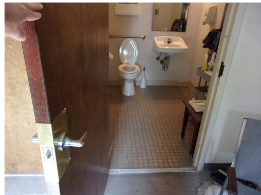
555 West Bay Street Office - Women's staff restroom - Replace common restroom accessories (Non-Critical Repair)
