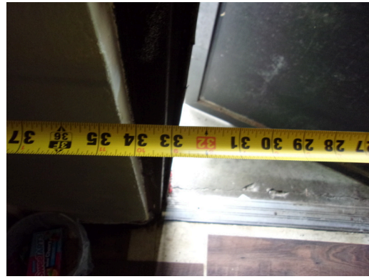
260-268 Yamacraw Village - Unit 261 - 1-bed/ 1-bath - HC unit - 32 inch clear opening at front door
