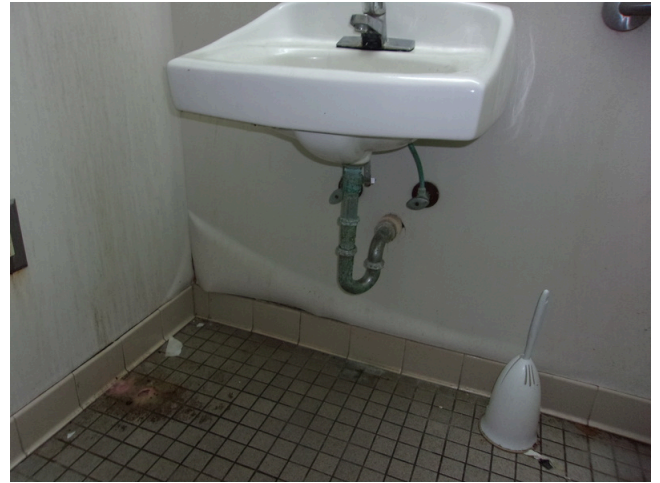
70. 555 West Bay Street Office - Men's staff restroom - No scald and abrasion protection (Critical Repair)
