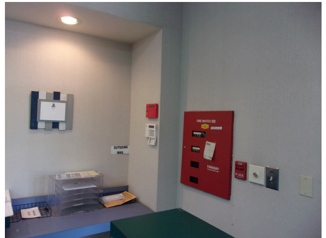
144. 555 West Bay Street Office - Fire alarm - Provide annual report (Critical Repair)
