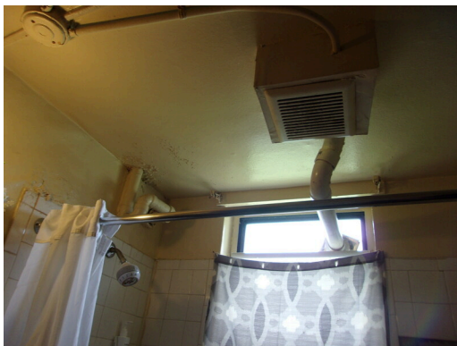
260-268 Yamacraw Village - Unit 261 - 1-bed/ 1-bath - HC unit - Direct vent bath fan
