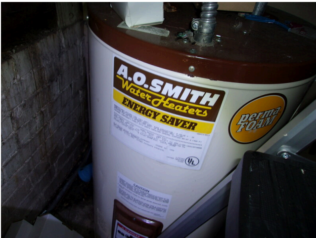
147. 555 West Bay Street Office - Replace old 20-gallon water heater (Non-Critical Repair)
