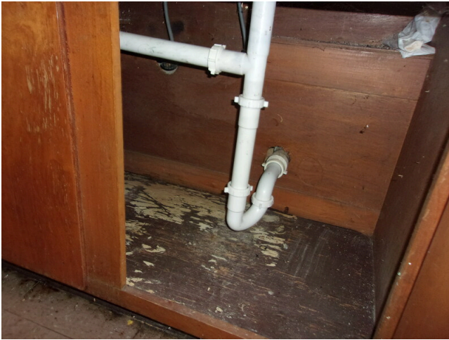
9. 121-128 Yamacraw Village - Unit 126 - 2-bed/ 1-bath TH - PVC waste pipe
