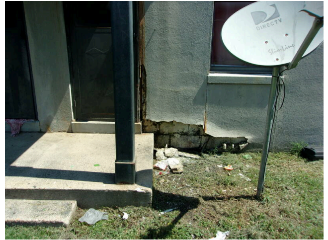
38. Damaged stucco siding near rear entry door (Non-Critical Repair)
