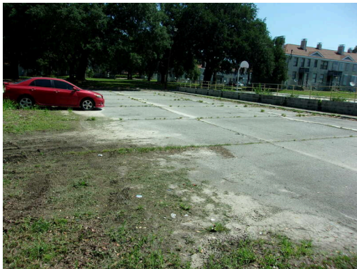
Replace asphalt parking lot and restripe (Non-Critical Repair)
