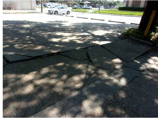
Replace heaving and cracked concrete parking lot (Non-Critical Repair)
