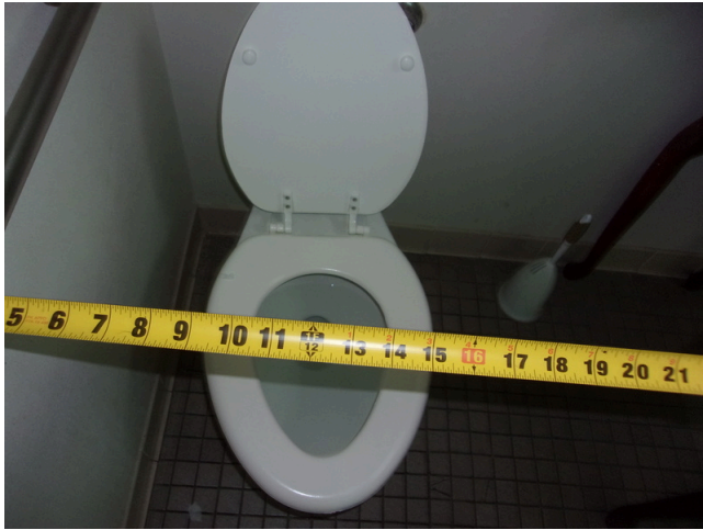
77. 555 West Bay Street Office - Women's public restroom - Move toilet to 18 inches from centerline to side wall (Critical Repair)
