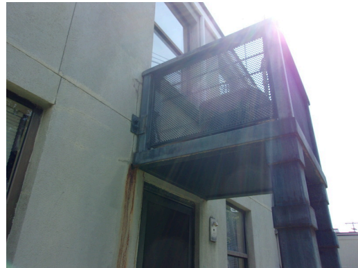
Replace metal AC canopies, rusting and causing water infiltration issues (Non-Critical Repair)
