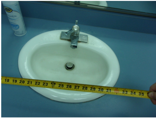
555 West Bay Street Office - Women's public restroom - Clear floor space at sink
