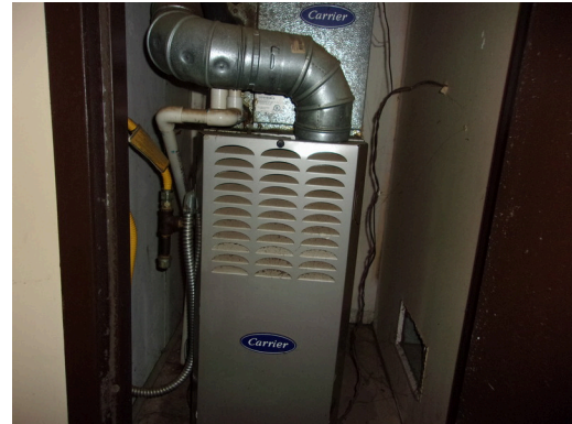
141-148 Yamacraw Village - Unit 142 - 3-bed/ 1-bath TH - Replace old gas furnace (Non-Critical Repair)
