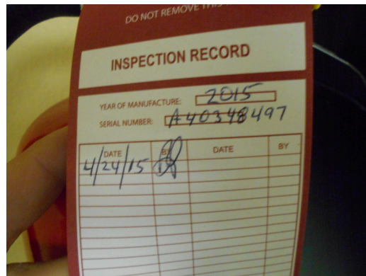
349 West Bryan Street - Community center - Inspect fire extinguishers annually (Critical Repair)
