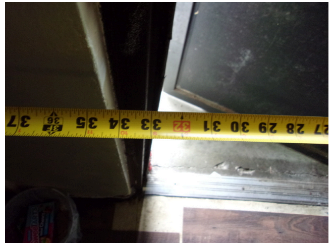
32. 260-268 Yamacraw Village - Unit 261 - 1-bed/ 1-bath - HC unit - 32 inch clear opening at front door
