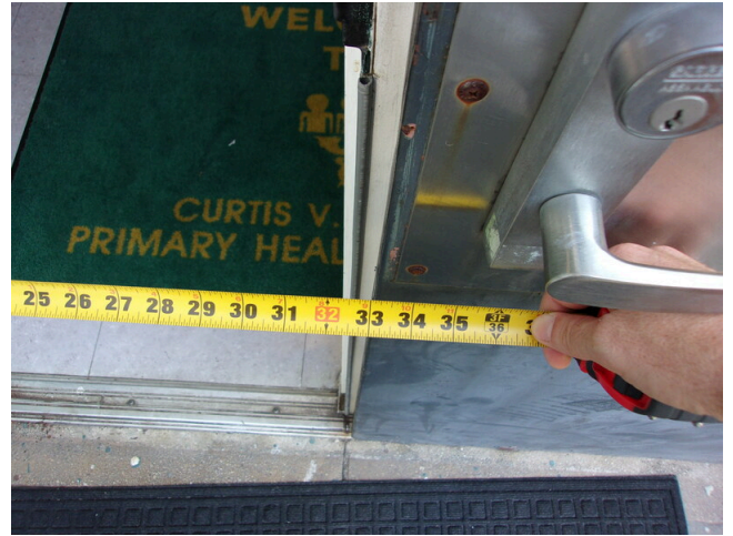
102. 349 West Bryan Street - 2nd floor Doctor's office - 32 inch clear opening at door
