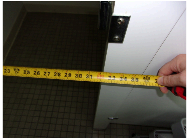
76. 555 West Bay Street Office - Women's public restroom - 32 inch clear opening at HC stall door
