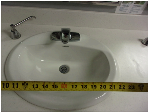
349 West Bryan Street - 2nd floor Doctor's office - Men's public restroom - Clear floor space at sinks
