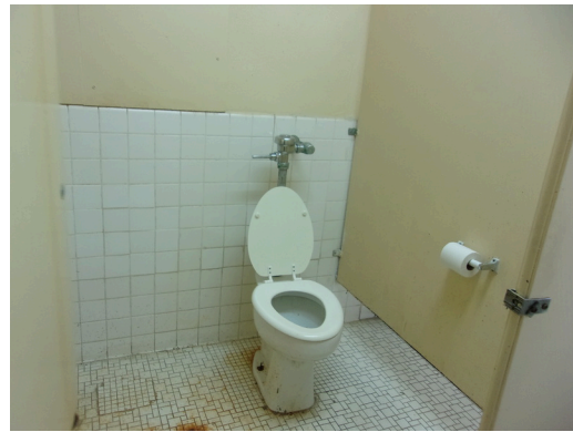
349 West Bryan Street - Community center - Men's restroom - Replace common restrooms accessories (Non-Critical Repair)
