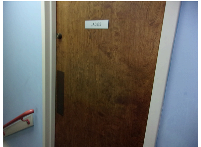
72. 555 West Bay Street Office - Women's public restroom - No ADA signage (Critical Repair)
