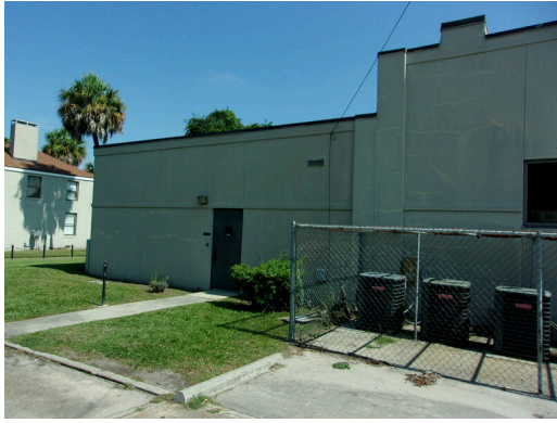
Chain link HVAC fencing
