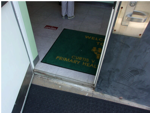
349 West Bryan Street - 2nd floor Doctor's office - Low threshold at main entry door
