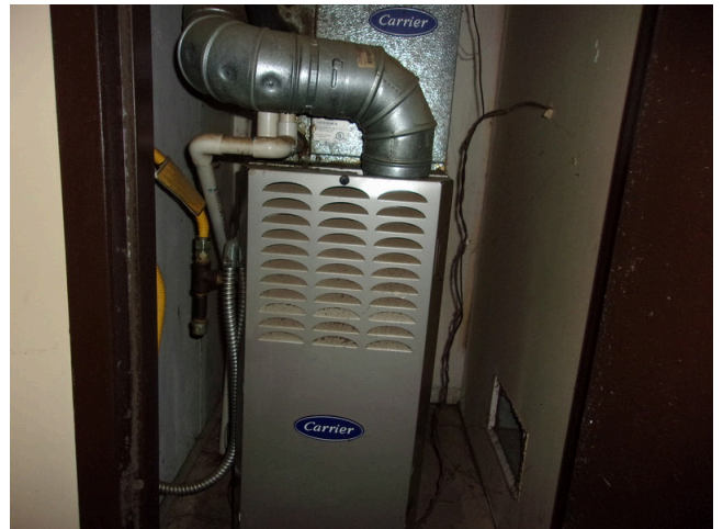
24. 141-148 Yamacraw Village - Unit 142 - 3-bed/ 1-bath TH - Replace old gas furnace (Non-Critical Repair)
