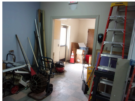
555 West Bay Street Office - Maintenance areas - Replace old vinyl flooring (Non-Critical Repair)
