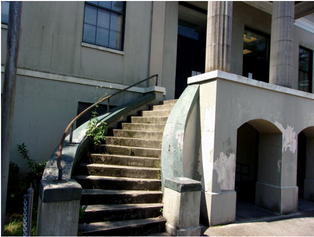
45. Replace deteriorating concrete steps at 349 West Bryan Street (Non-Critical Repair)
