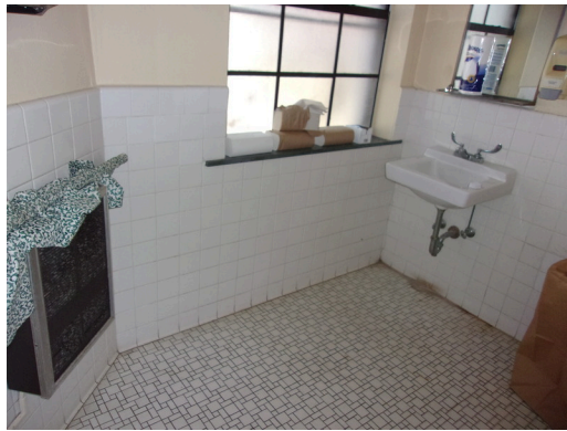
349 West Bryan Street - Community center - Women's restroom - Install scald and abrasion protection (Critical Repair)
