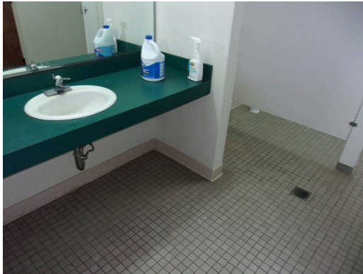
555 West Bay Street Office - Men's public restroom - Replace common restroom accessories (Non-Critical Repair)
