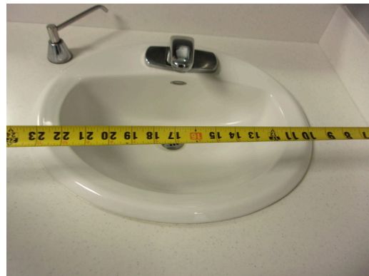
349 West Bryan Street - 2nd floor Doctor's office - Women's public restroom - Clear floor space at sinks
