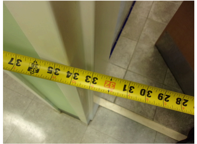
110. 349 West Bryan Street - 2nd floor Doctor's office - Men's public restroom - 32 inch clear opening
