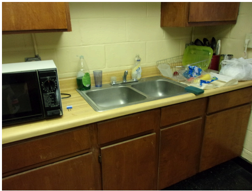
349 West Bryan Street - Community center - Common kitchen - Replace old kitchen cabinetry (Non-Critical Repair)
