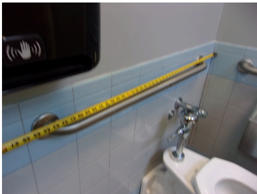
349 West Bryan Street - 2nd floor Doctor's office - Women's public restroom - Compliant rear grab bar
