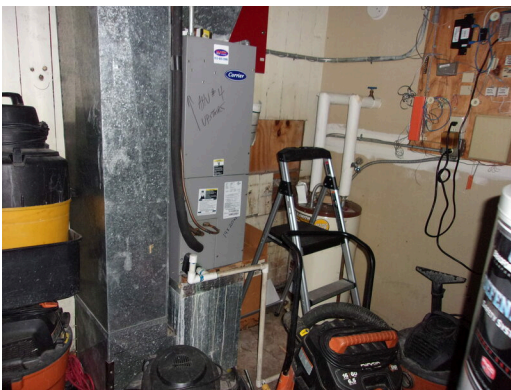
555 West Bay Street Office - Mechanical room with AHU and electric water heater
