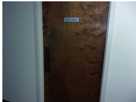
555 West Bay Street Office - Men's public restroom - No ADA signage (Critical Repair)
