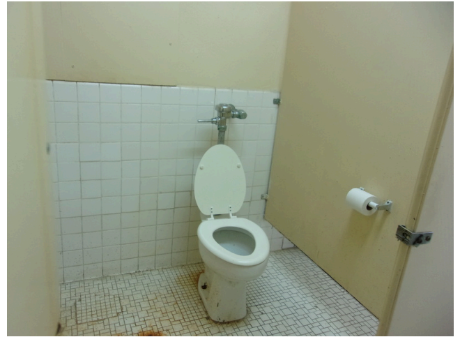
142. 349 West Bryan Street - Community center - Men's restroom - Replace common restrooms accessories (Non-Critical Repair)
