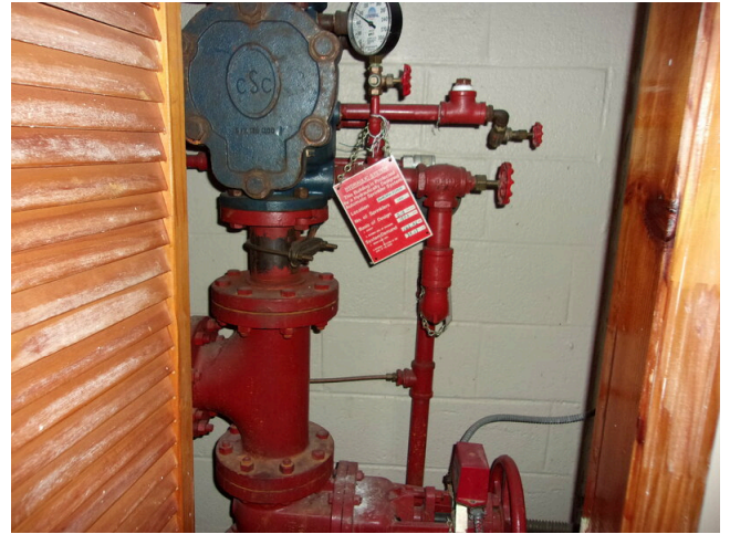
150. 349 West Bryan Street - Community center - Fire riser - Provide annual sprinkler report (Critical Repair)
