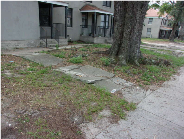
5. Typical damaged concrete sidewalk with trip hazards (Critical Repair)
