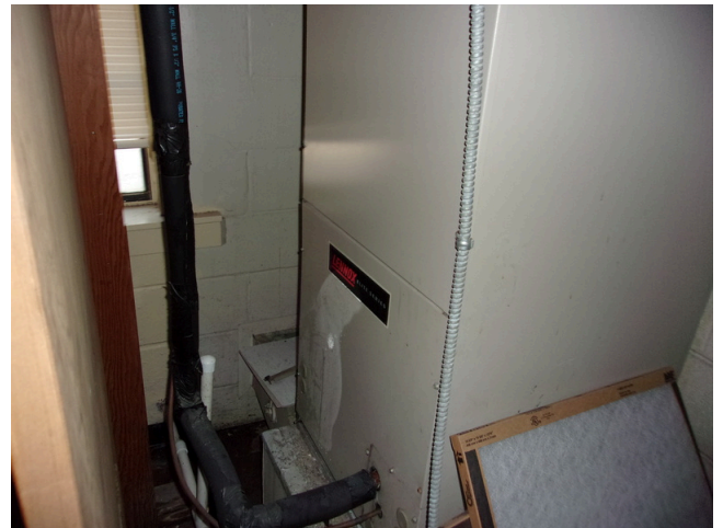
152. 349 West Bryan Street - Community center - Air handler
