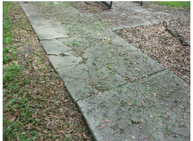
4. Typical damaged concrete sidewalk with trip hazards (Critical Repair)
