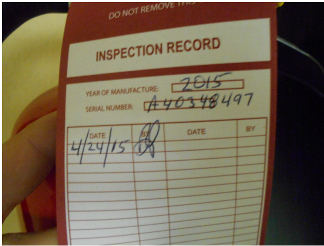
165. 349 West Bryan Street - Community center - Inspect fire extinguishers annually (Critical Repair)
