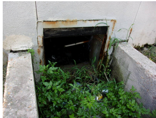
Broken plumbing pipe within crawlspace (Non-Critical Repair)
