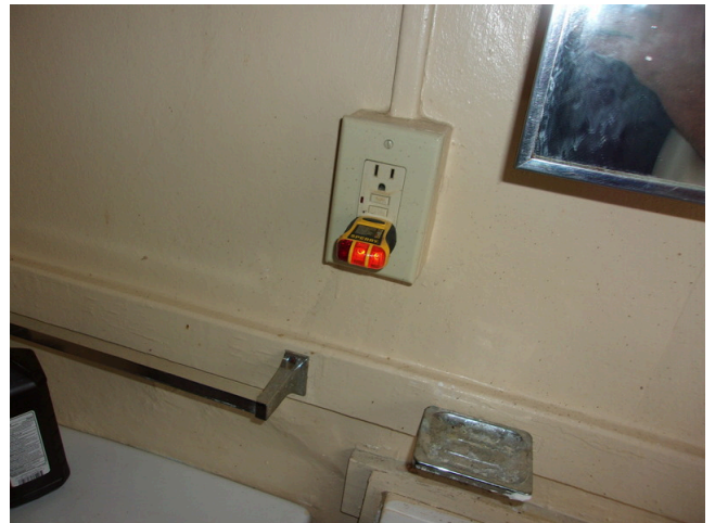
16. 121-128 Yamacraw Village - Unit 126 - 2-bed/ 1-bath TH - GFCI in bathroom
