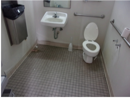
555 West Bay Street Office - Men's staff restroom - Replace common restroom accessories (Non-Critical Repair)
