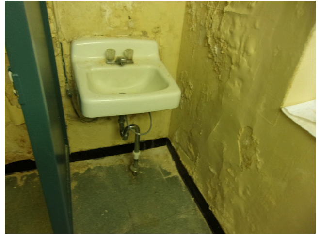
134. 349 West Bryan Street - Community center - Staff restroom with no scald and abrasion at the sink (Critical Repair)
