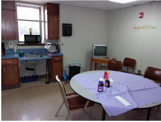
555 West Bay Street Office - Common staff kitchen - Replace kitchen cabinetry (Non-Critical Repair)
