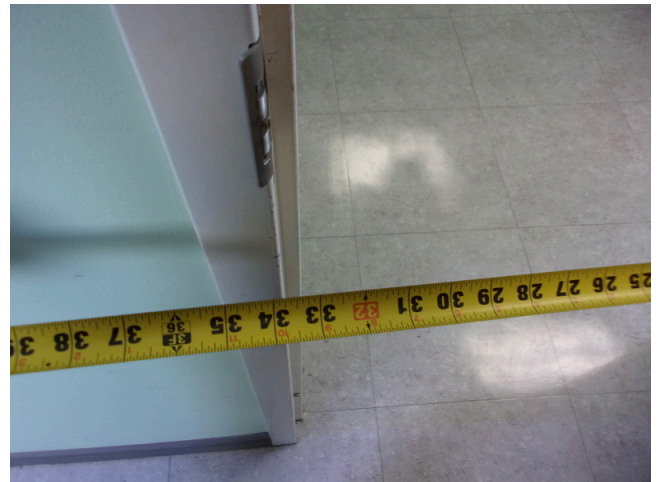
104. 349 West Bryan Street - 2nd floor Doctor's office - 33 inch clear opening to exam rooms
