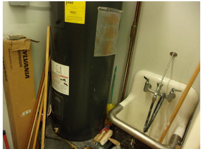
148. 349 West Bryan Street - 2nd floor Doctor's office - Mechanical room with water heater
