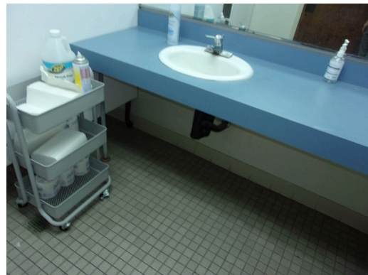
555 West Bay Street Office - Women's public restroom - Levered sink with scald and abrasion protection, replace common restroom accessories (Non-Critical Repair)
