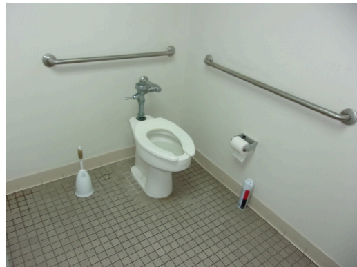
555 West Bay Street Office - Men's public restroom - Toilet with compliant grab bars
