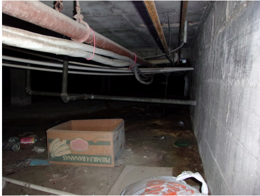
View of plumbing/gas pipe and electrical wiring in crawlspace
