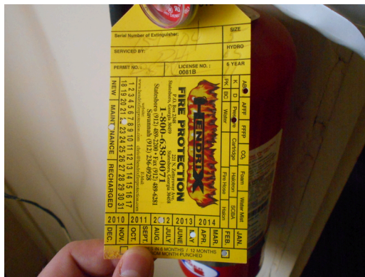
349 West Bryan Street - Community center - Inspect fire extinguishers annually (Critical Repair)
