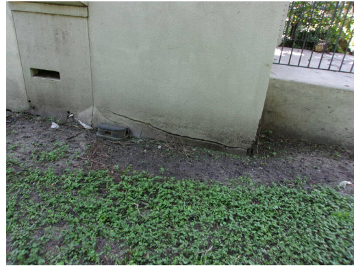
Evidence of foundation settling, damaged stucco siding (Non-Critical Repair)
