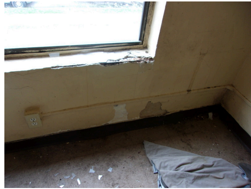
260-268 Yamacraw Village - Unit 264 - 2-bed/ 1-bath TH - Plaster wall damage (Non-Critical Repair)
