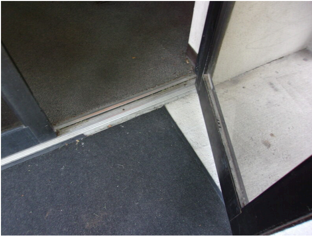
61. 555 West Bay Street Office - Low threshold at main entry doors
