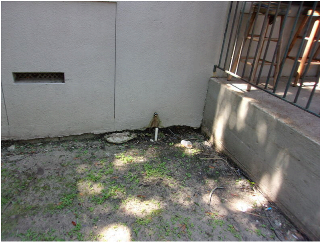
33. Damaged stucco siding (Non-Critical Repair)
