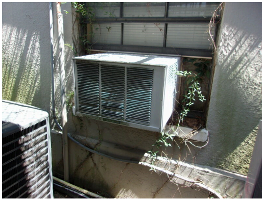
Window AC unit
