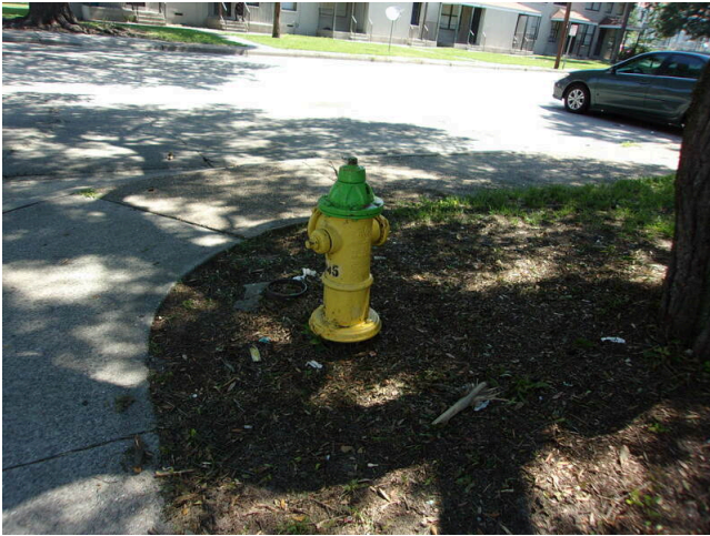
157. Fire hydrant near municipal street
