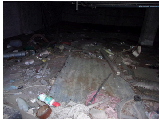
Crawlspace floor without vapor barrier
