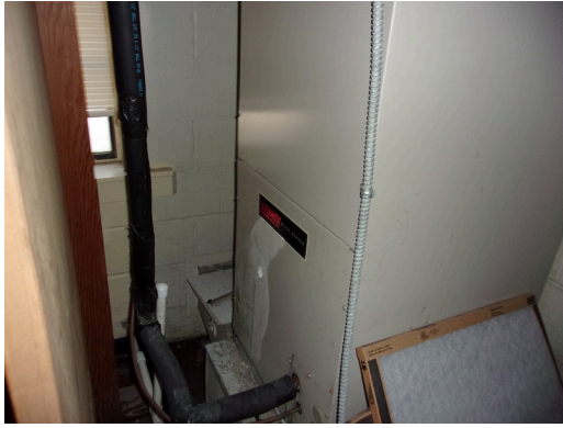
349 West Bryan Street - Community center - Air handler
