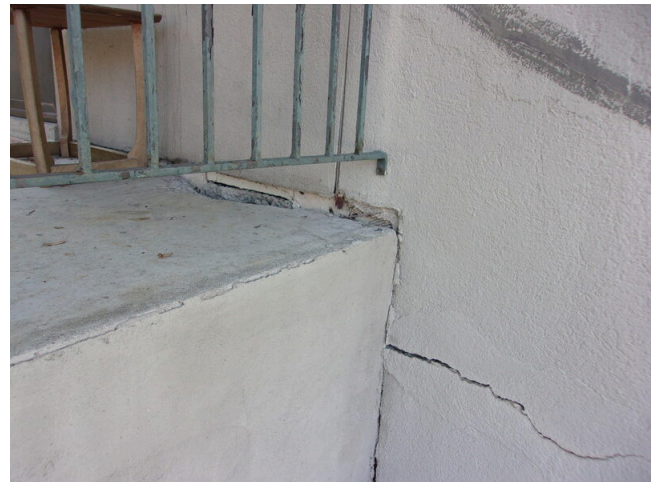
40. Front porch sinking (Non-Critical Repair)
