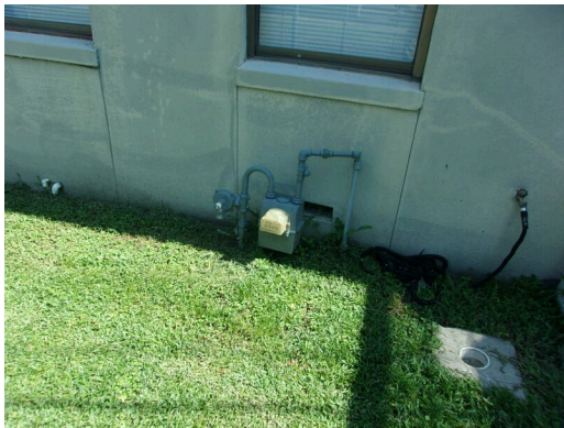
Typical gas meter
