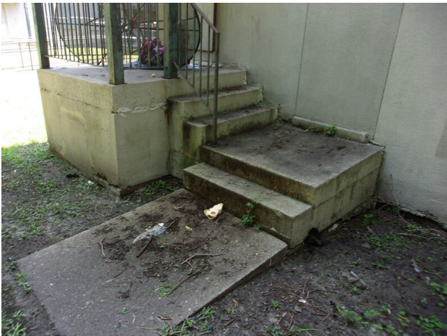
27. Sinking porch steps (Non-Critical Repair)
