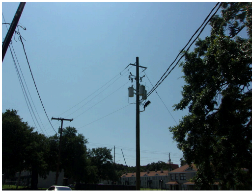
Pole mounted transformers
