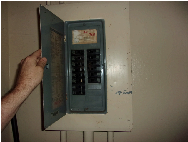
21. 141-148 Yamacraw Village - Unit 142 - 3-bed/ 1-bath TH - Breaker panel
