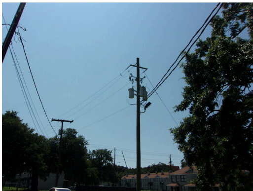
Pole mounted transformers
