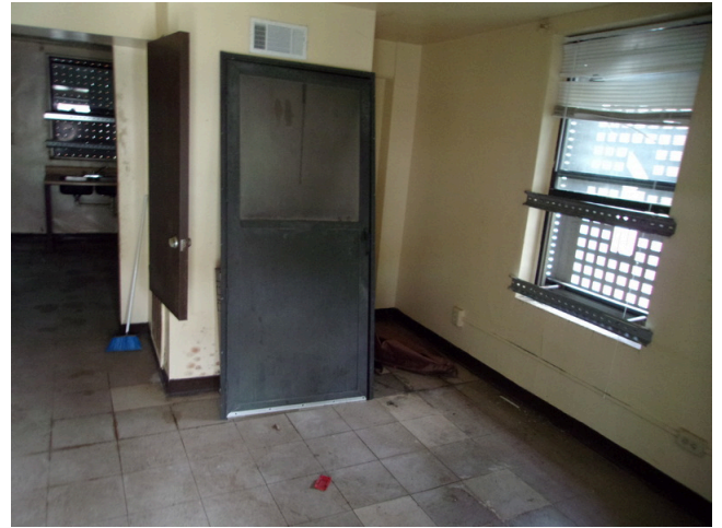
66. 460-467 Yamacraw Village - Unit 461 - 1-bed/ 1-bath - HC unit/Down unit - Living room view, replace flooring (Non-Critical Repair)
