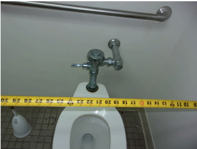
87. 555 West Bay Street Office - Men's public restroom - Clear floor space at toilet
