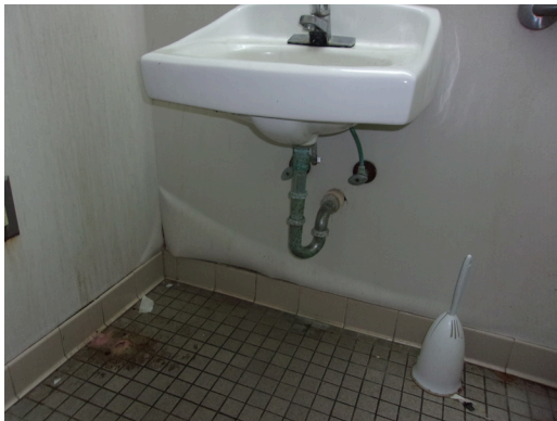
555 West Bay Street Office - Men's staff restroom - No scald and abrasion protection (Critical Repair)
