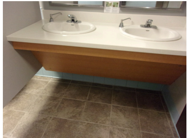
124. 349 West Bryan Street - 2nd floor Doctor's office - Women's public restroom - Scald and abrasion protection at sinks
