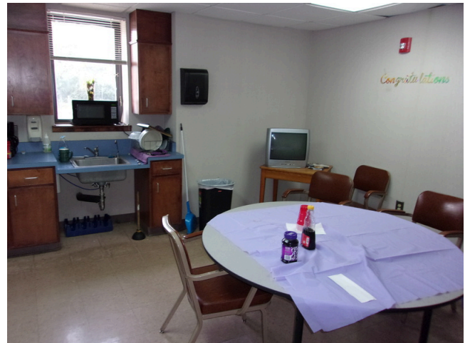
88. 555 West Bay Street Office - Common staff kitchen - Replace kitchen cabinetry (Non-Critical Repair)
