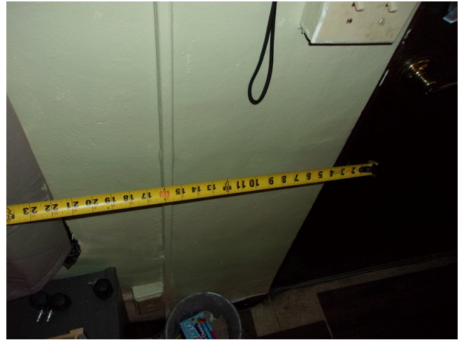
34. 260-268 Yamacraw Village - Unit 261 - 1-bed/ 1-bath - HC unit - Adequate space at latch side of door
