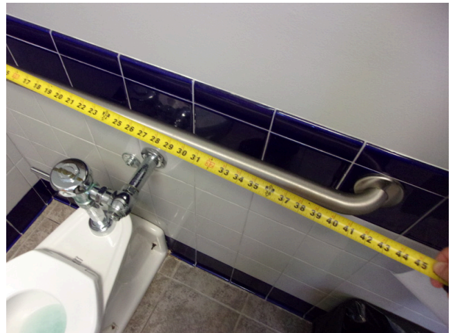
116. 349 West Bryan Street - 2nd floor Doctor's office - Men's public restroom - Compliant rear grab bar
