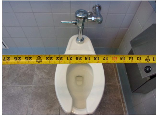
126. 349 West Bryan Street - 2nd floor Doctor's office - Women's public restroom - Clear floor space at toilet
