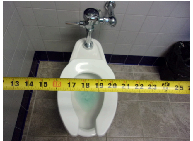
114. 349 West Bryan Street - 2nd floor Doctor's office - Men's public restroom - Clear floor space at toilet
