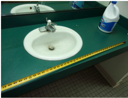
555 West Bay Street Office - Men's public restroom - Clear floor space at levered sink
