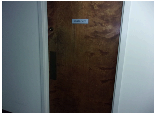
80. 555 West Bay Street Office - Men's public restroom - No ADA signage (Critical Repair)
