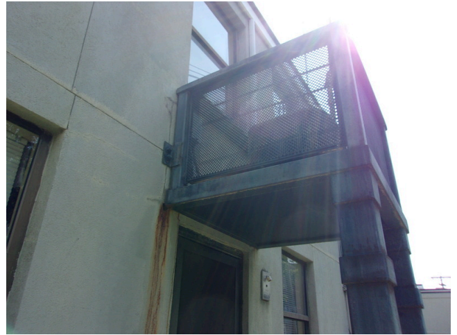
18. Replace metal AC canopies, rusting and causing water infiltration issues (Non-Critical Repair)
