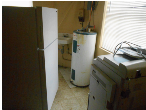
349 West Bryan Street - Community center - Replace old 50-gallon water heater (Non-Critical Repair)
