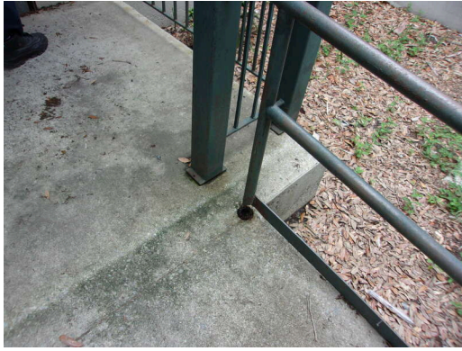
Replace concrete and metal HC unit ramps (Non-Critical Repair)
