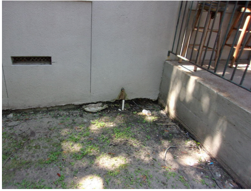
Damaged stucco siding (Non-Critical Repair)
