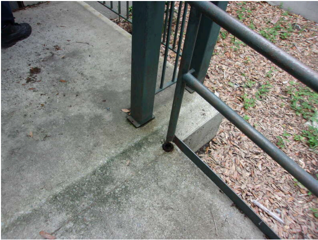
53. Replace concrete and metal HC unit ramps (Non-Critical Repair)
