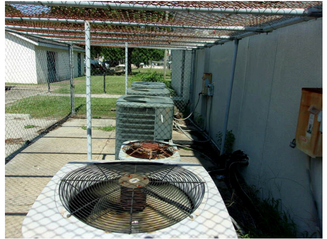
154. Heat pump condenser units
