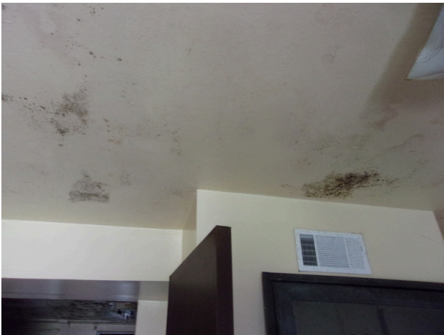
67. 460-467 Yamacraw Village - Unit 461 - 1-bed/ 1-bath - HC unit/Down unit - Mold growth throughout (Non-Critical Repair)
