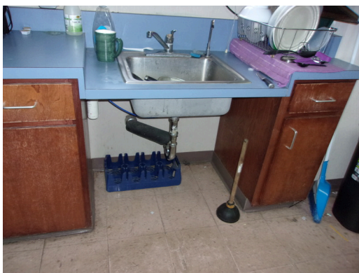
555 West Bay Street Office - No scald and abrasion protection at kitchen sink (Critical Repair)
