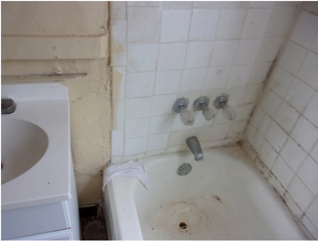
17. 121-128 Yamacraw Village - Unit 126 - 2-bed/ 1-bath TH - Replace ceramic tile surround (Non- Critical Repair)
