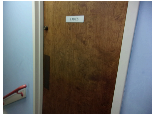
555 West Bay Street Office - Women's public restroom - No ADA signage (Critical Repair)
