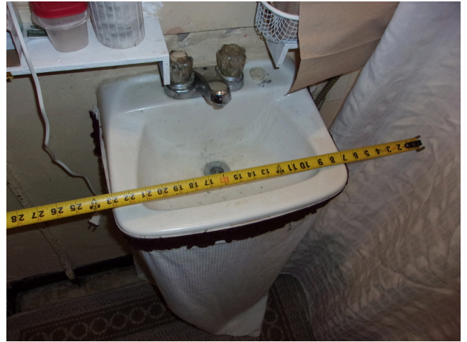
50. 260-268 Yamacraw Village - Unit 261 - 1-bed/ 1-bath - HC unit - Clear floor space at roll-under sink
