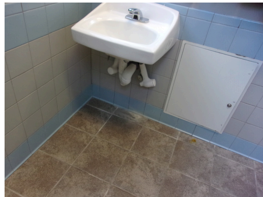
349 West Bryan Street - 2nd floor Doctor's office - Women's public restroom - Scald and abrasion protection at sink
