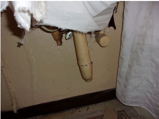
51. 260-268 Yamacraw Village - Unit 261 - 1-bed/ 1-bath - HC unit - Partial scald and abrasion at sink
