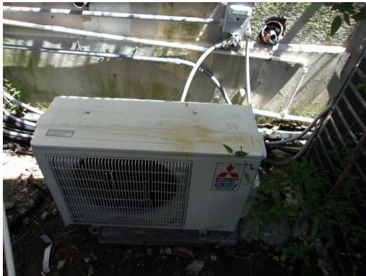
349 West Bryan Street - Mini-split unit
