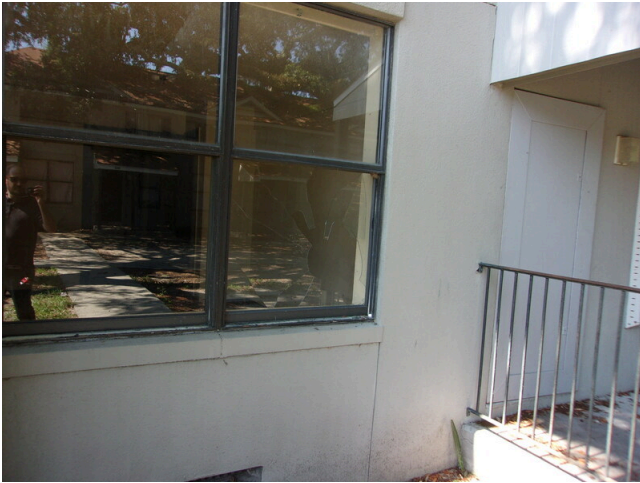
29. Typical broken window (Non-Critical Repair)
