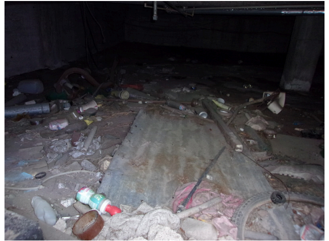
94. Crawlspace floor without vapor barrier
