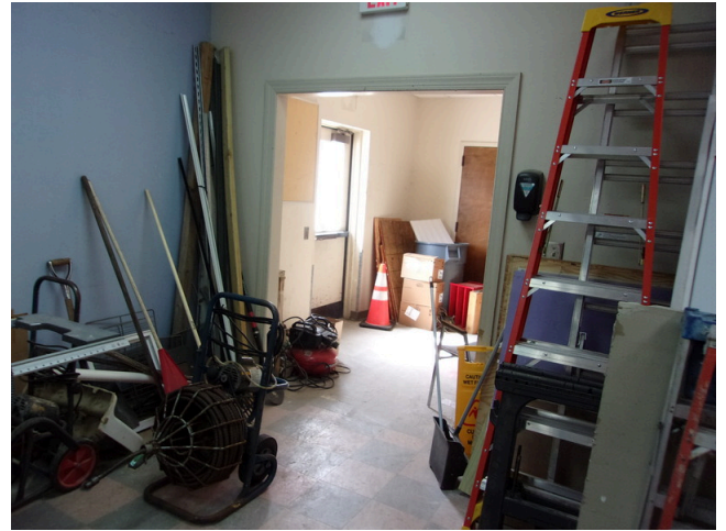
66. 555 West Bay Street Office - Maintenance areas - Replace old vinyl flooring (Non-Critical Repair)
