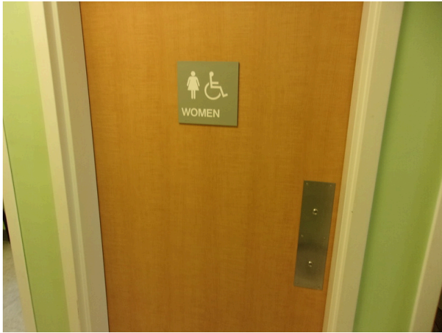
121. 349 West Bryan Street - 2nd floor Doctor's office - Women's public restroom - ADA signage
