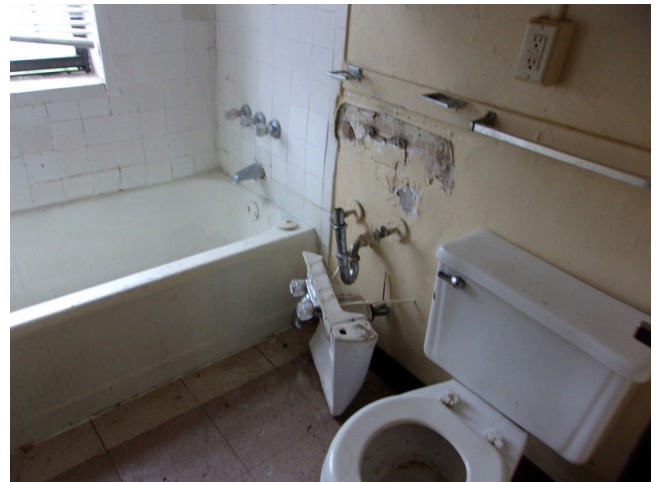
64. 260-268 Yamacraw Village - Unit 264 - 2-bed/ 1-bath TH - Damaged plumbing fixtures and plaster wall (Non-Critical Repair)
