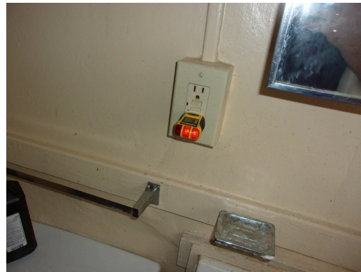
121-128 Yamacraw Village - Unit 126 - 2-bed/ 1-bath TH - GFCI in bathroom
