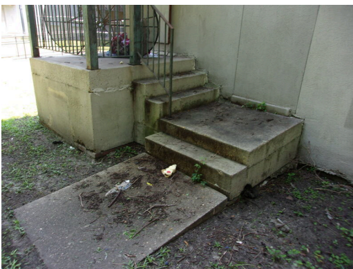
Sinking porch steps (Non-Critical Repair)
