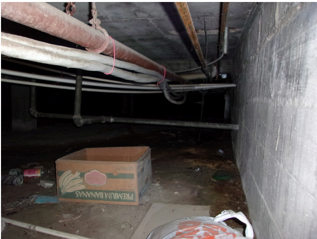
95. View of plumbing/gas pipe and electrical wiring in crawlspace
