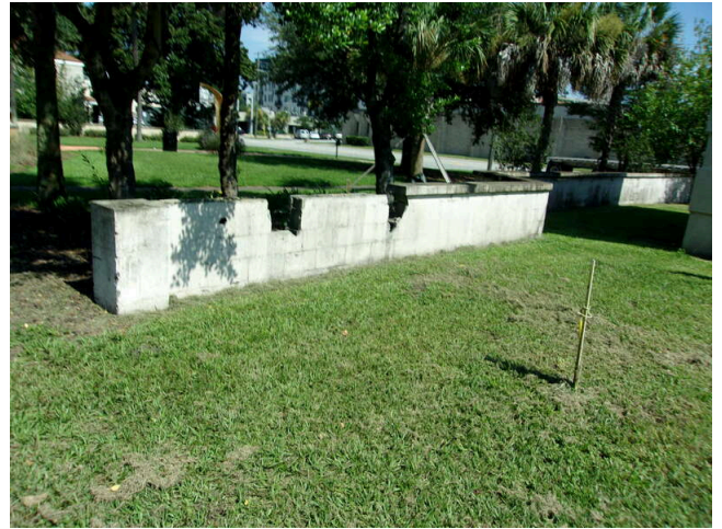
22. Replace damaged CMU retaining walls (Non-Critical Repair)
