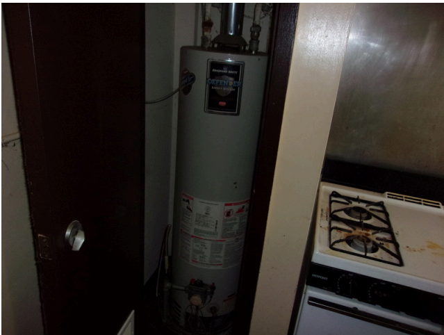
11. 121-128 Yamacraw Village - Unit 126 - 2-bed/ 1-bath TH - Replace gas-fired water heater (Non- Critical Repair)
