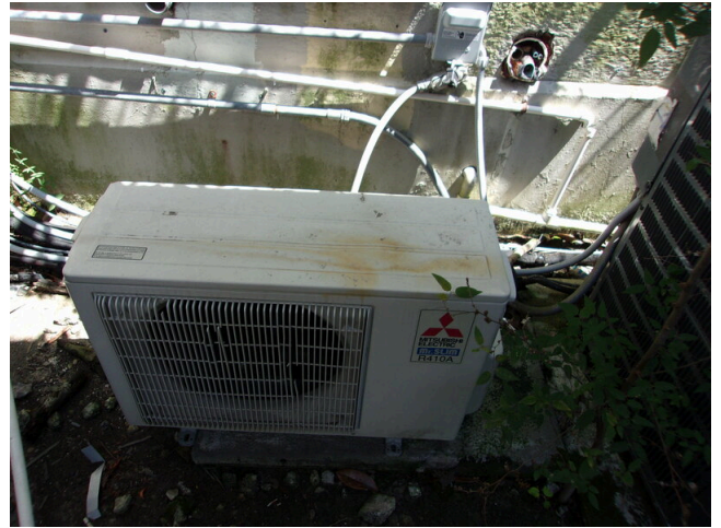
162. 349 West Bryan Street - Mini-split unit
