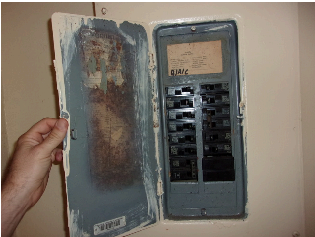
7. 121-128 Yamacraw Village - Unit 126 - 2-bed/ 1-bath TH - Breaker panel
