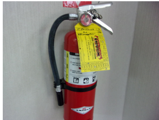
555 West Bay Street Office - Fire extinguisher - Tag dated July 2023
