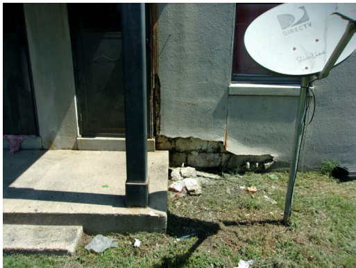
Damaged stucco siding near rear entry door (Non-Critical Repair)
