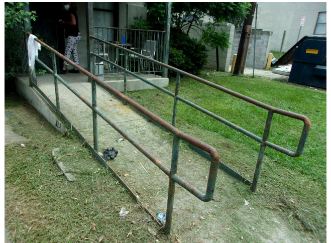
52. Replace concrete and metal HC unit ramps (Non-Critical Repair)
