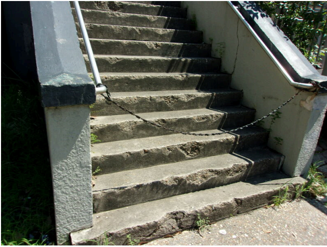
49. 349 West Bryan Street - Replace steep and deteriorating concrete steps at rear (Non-Critical Repair)
