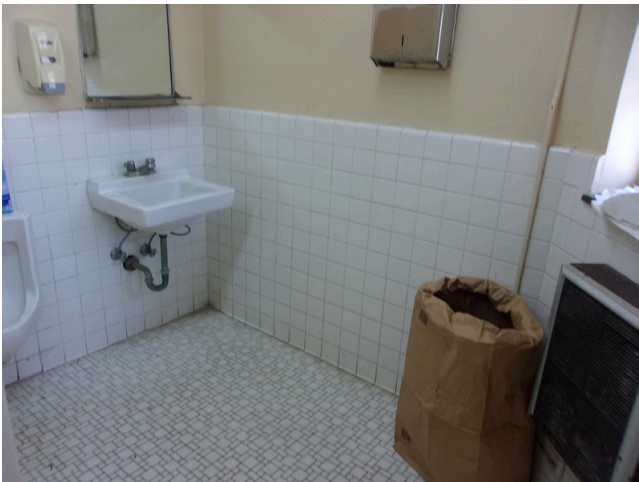
143. 349 West Bryan Street - Community center - Men's restroom - Install scald and abrasion protection (Critical Repair)
