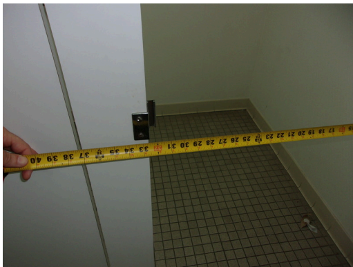
555 West Bay Street Office - Men's public restroom - 32 inch clear opening at HC stall door
