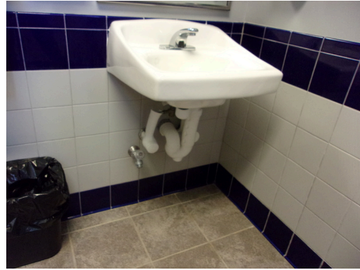
349 West Bryan Street - 2nd floor Doctor's office - Men's public restroom - Scald and abrasion at sink
