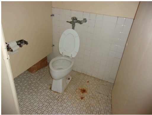
349 West Bryan Street - Community center - Women's restroom - Replace common restroom accessories (Non-Critical Repair)
