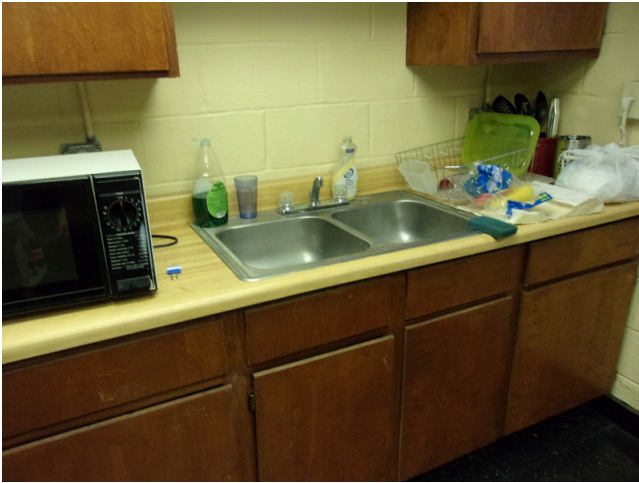
137. 349 West Bryan Street - Community center - Common kitchen - Replace old kitchen cabinetry (Non-Critical Repair)
