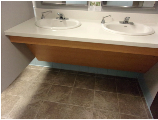
349 West Bryan Street - 2nd floor Doctor's office - Women's public restroom - Scald and abrasion protection at sinks
