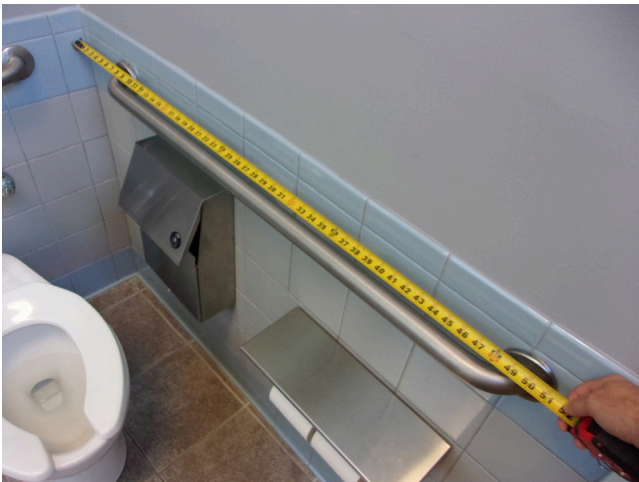
127. 349 West Bryan Street - 2nd floor Doctor's office - Women's public restroom - Compliant side grab bar
