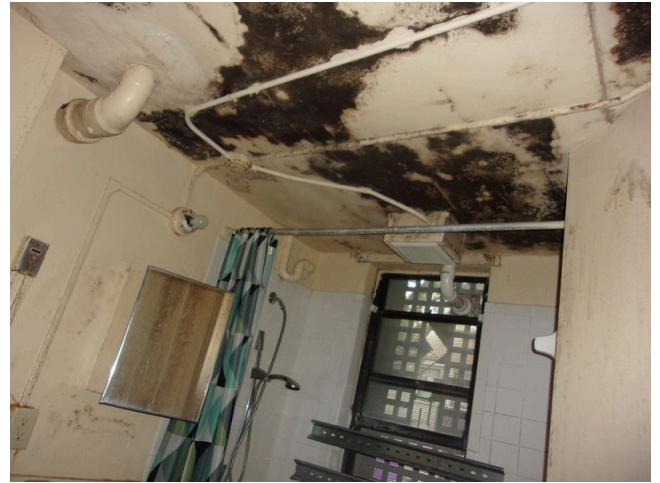
70. 460-467 Yamacraw Village - Unit 461 - 1-bed/ 1-bath - HC unit/Down unit - Mold growth throughout (Non-Critical Repair)
