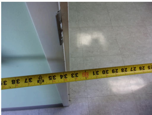
349 West Bryan Street - 2nd floor Doctor's office - 33 inch clear opening to exam rooms
