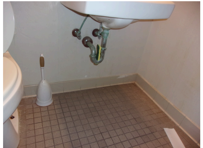
68. 555 West Bay Street Office - Women's restroom - No scald and abrasion protection (Critical Repair)
