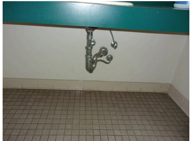
84. 555 West Bay Street Office - Men's public restroom - No scald and abrasion protection at sink (Critical Repair)
