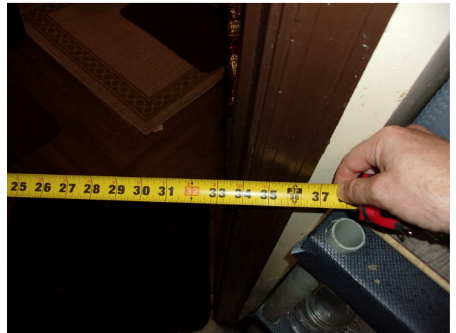
48. 260-268 Yamacraw Village - Unit 261 - 1-bed/ 1-bath - HC unit - 32 inch clear opening at bathroom door
