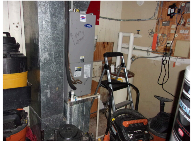
146. 555 West Bay Street Office - Mechanical room with AHU and electric water heater
