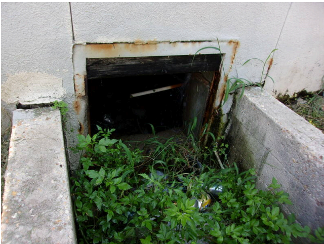
31. Broken plumbing pipe within crawlspace (Non-Critical Repair)
