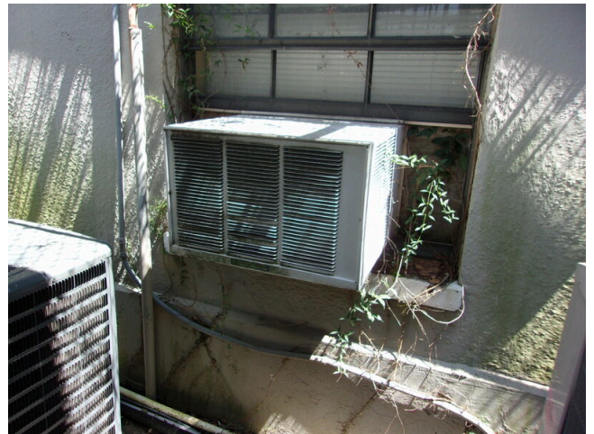
160. Window AC unit
