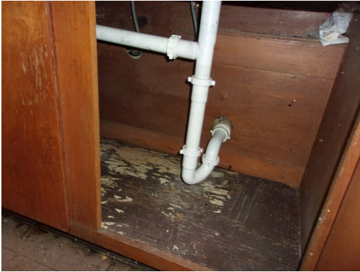
121-128 Yamacraw Village - Unit 126 - 2-bed/ 1-bath TH - PVC waste pipe
