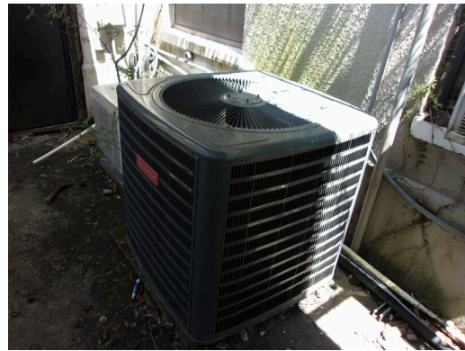
349 West Bryan Street - Heat pump unit
