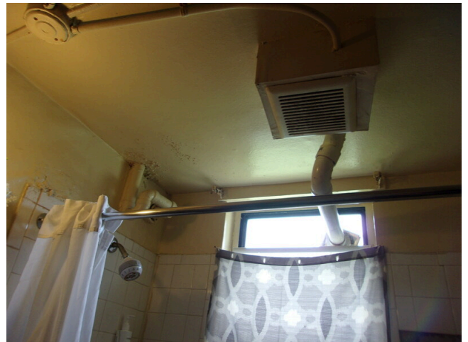
52. 260-268 Yamacraw Village - Unit 261 - 1-bed/ 1-bath - HC unit - Direct vent bath fan
