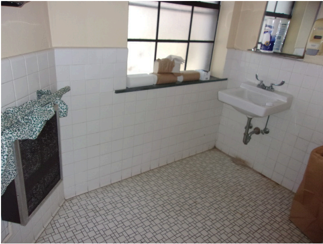
141. 349 West Bryan Street - Community center - Women's restroom - Install scald and abrasion protection (Critical Repair)
