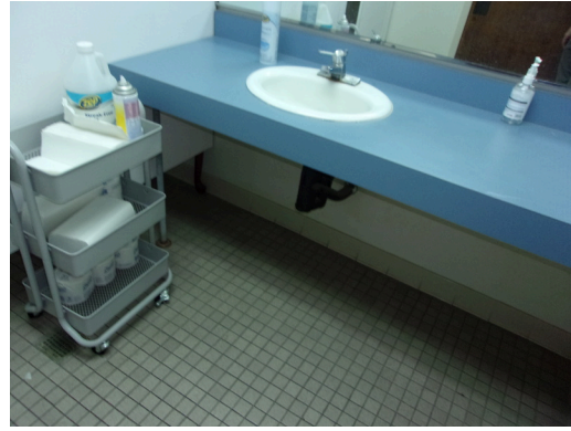
555 West Bay Street Office - Women's public restroom - Levered sink with scald and abrasion protection, replace common restroom accessories (Non-Critical Repair)
