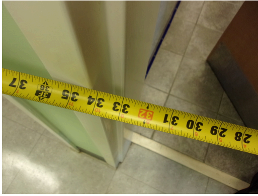
349 West Bryan Street - 2nd floor Doctor's office - Men's public restroom - 32 inch clear opening
