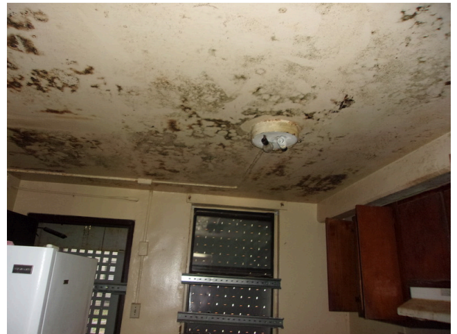
68. 460-467 Yamacraw Village - Unit 461 - 1-bed/ 1-bath - HC unit/Down unit - Mold growth throughout (Non-Critical Repair)
