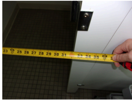
555 West Bay Street Office - Women's public restroom - 32 inch clear opening at HC stall door
