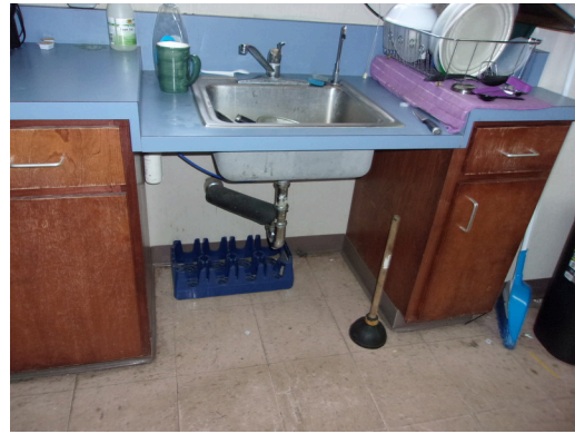
555 West Bay Street Office - No scald and abrasion protection at kitchen sink (Critical Repair)
