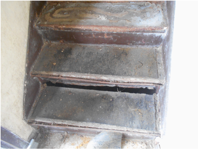
73. 460-467 Yamacraw Village - Unit 460 - 1-bed/ 1-bath - Down unit - Replace damaged interior stairs (Non-Critical Repair)
