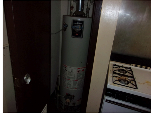
121-128 Yamacraw Village - Unit 126 - 2-bed/ 1-bath TH - Replace gas-fired water heater (Non-Critical Repair)
