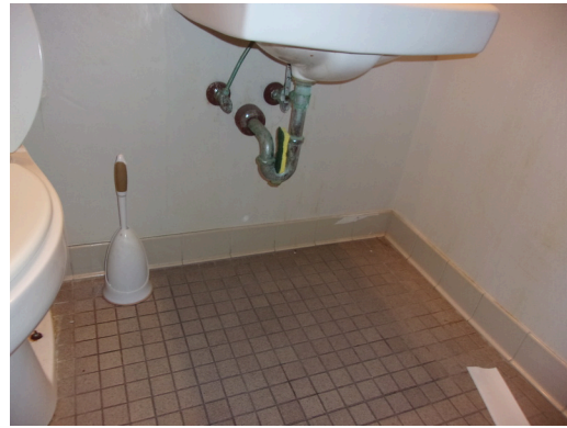
555 West Bay Street Office - Women's restroom - No scald and abrasion protection (Critical Repair)
