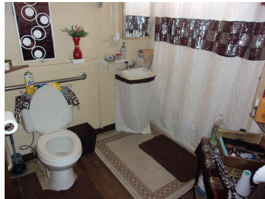
260-268 Yamacraw Village - Unit 261 - 1-bed/ 1-bath - HC unit - Bathroom view, toilet with grab bars
