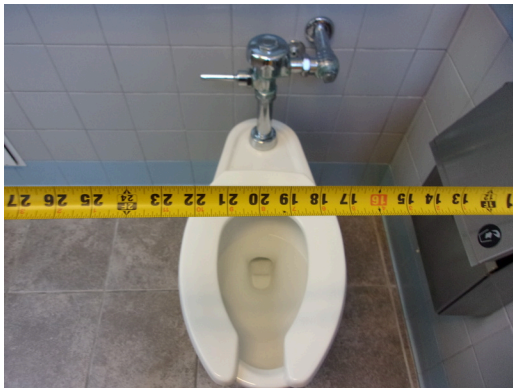
349 West Bryan Street - 2nd floor Doctor's office - Women's public restroom - Clear floor space at toilet
