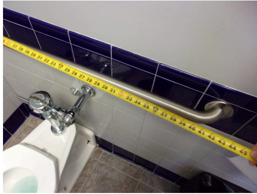
349 West Bryan Street - 2nd floor Doctor's office - Men's public restroom - Compliant rear grab bar
