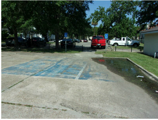
HC parking at 555 West Bay Street - Two (2) standard spaces, convert two (2) spaces to van accessible (Critical Repair)
