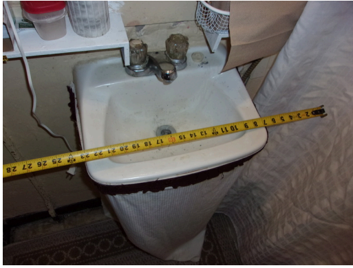
260-268 Yamacraw Village - Unit 261 - 1-bed/ 1-bath - HC unit - Clear floor space at roll-under sink
