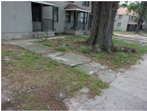
Typical damaged concrete sidewalk with trip hazards (Critical Repair)
