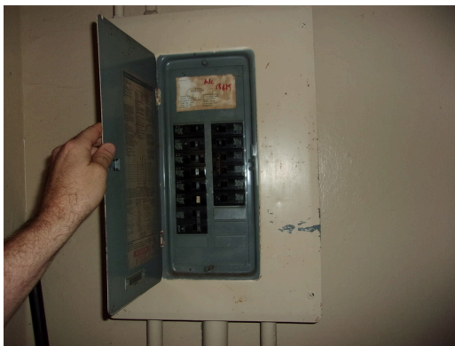
141-148 Yamacraw Village - Unit 142 - 3-bed/ 1-bath TH - Breaker panel
