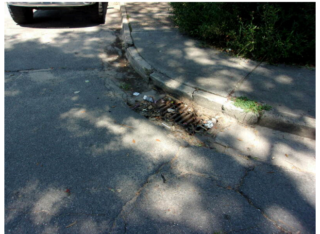
32. Municipal street storm water drain inlet
