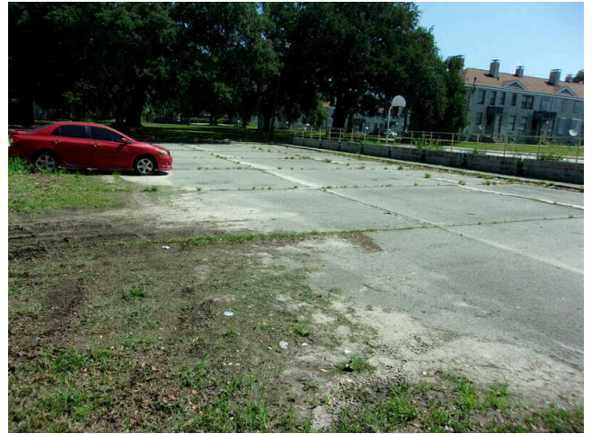
34. Replace asphalt parking lot and restripe (Non-Critical Repair)
