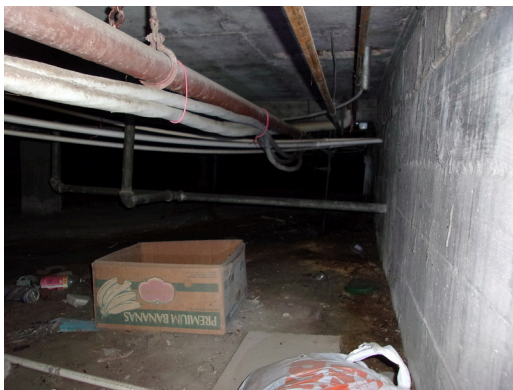
View of plumbing/gas pipe and electrical wiring in crawlspace
