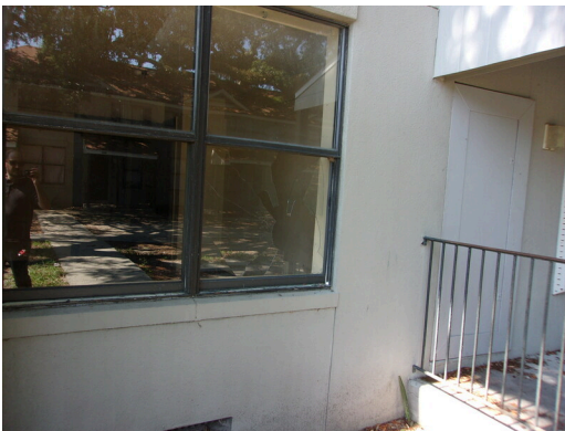
Typical broken window (Non-Critical Repair)
