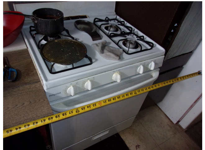
40. 260-268 Yamacraw Village - Unit 261 - 1-bed/ 1-bath - HC unit - Clear floor space at range/oven
