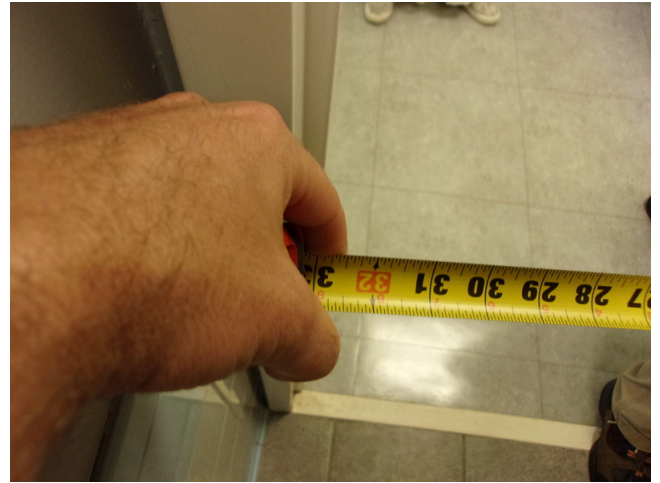
122. 349 West Bryan Street - 2nd floor Doctor's office - Women's public restroom - 33 inch clear opening at door
