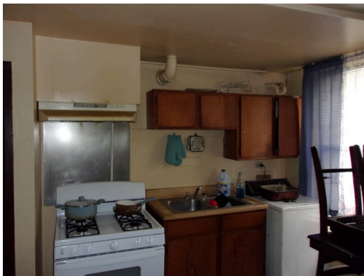
141-148 Yamacraw Village - Unit 142 - 3-bed/ 1-bath TH - Kitchen view, replace old cabinetry (Non-Critical Repair)
