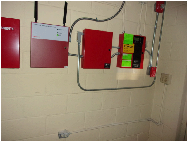
151. 349 West Bryan Street - Community center - Fire alarm panel - Provide annual report (Critical Repair)
