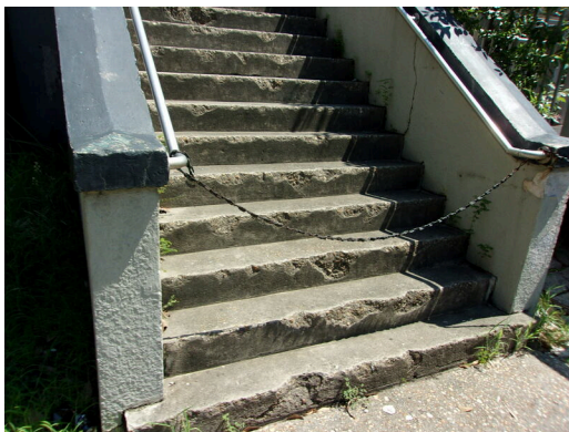
349 West Bryan Street - Replace steep and deteriorating concrete steps at rear (Non-Critical Repair)
