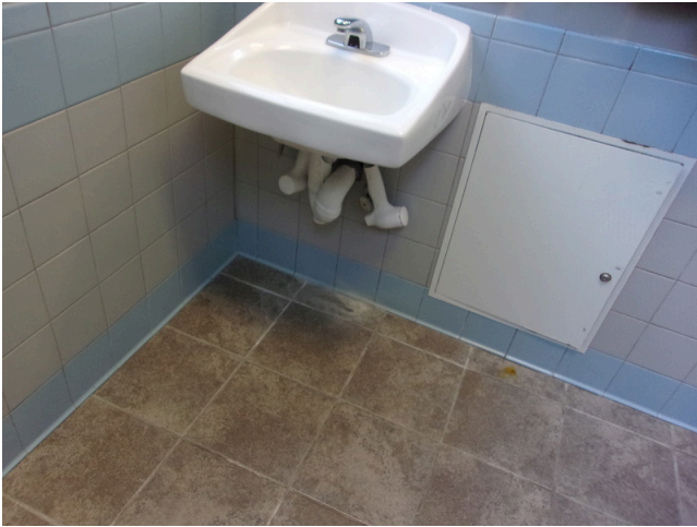
129. 349 West Bryan Street - 2nd floor Doctor's office - Women's public restroom - Scald and abrasion protection at sink
