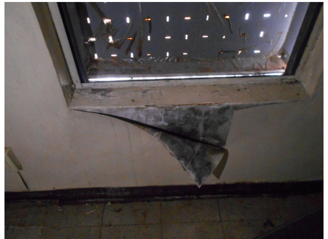
76. 460-467 Yamacraw Village - Unit 460 - 1-bed/ 1-bath - Down unit - Damaged plaster walls (Non- Critical Repair)
