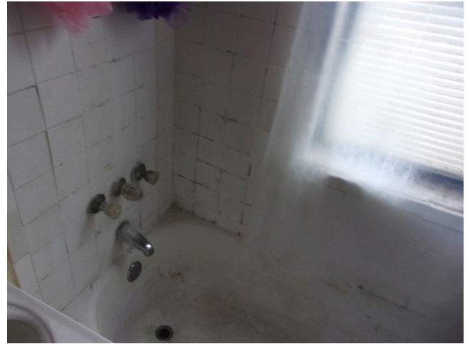
26. 141-148 Yamacraw Village - Unit 142 - 3-bed/ 1-bath TH - Replace damaged ceramic tile surround (Non-Critical Repair)
