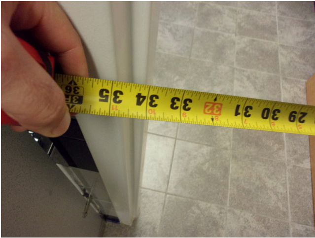
113. 349 West Bryan Street - 2nd floor Doctor's office - Men's public restroom - 34 inch clear opening at HC stall door
