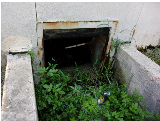
Broken plumbing pipe within crawlspace (Non-Critical Repair)
