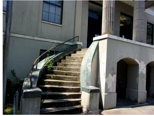
Replace deteriorating concrete steps at 349 West Bryan Street (Non-Critical Repair)
