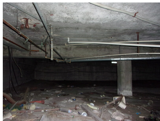
Spalling raised concrete slab (Non-Critical Repair), galvanized water supply lines
