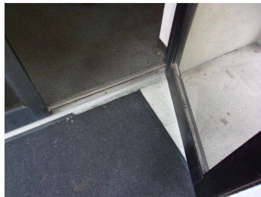
555 West Bay Street Office - Low threshold at main entry doors
