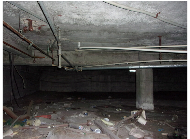
96. Spalling raised concrete slab (Non-Critical Repair), galvanized water supply lines
