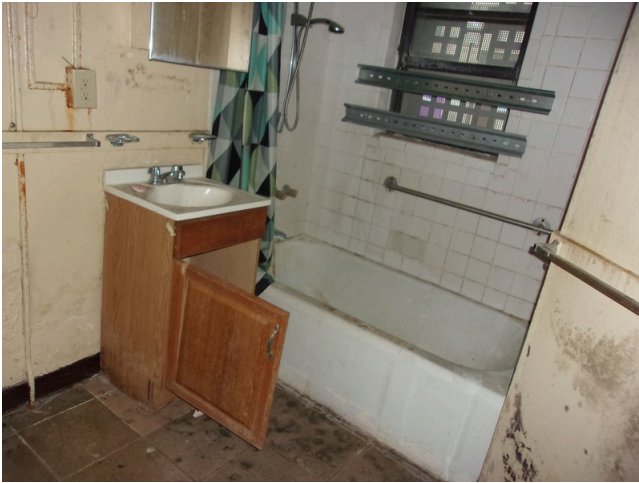
69. 460-467 Yamacraw Village - Unit 461 - 1-bed/ 1-bath - HC unit/Down unit - Mold growth throughout, replace plumbing fixtures and vanity (Non-Critical Repair)
