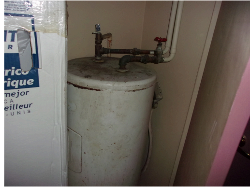
349 West Bryan Street - Community center - Replace old 50-gallon water heater (Non-Critical Repair)
