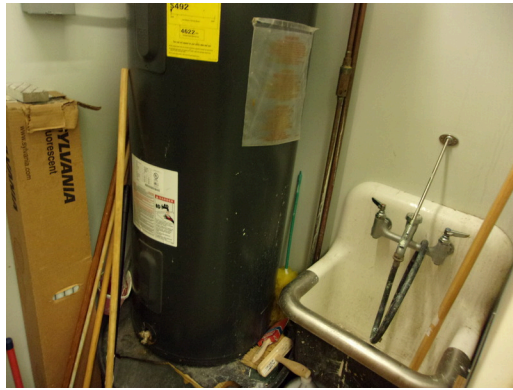
349 West Bryan Street - 2nd floor Doctor's office - Mechanical room with water heater
