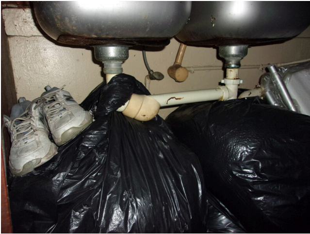
45. 260-268 Yamacraw Village - Unit 261 - 1-bed/ 1-bath - HC unit - No scald and abrasion at sink
