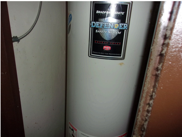
23. 141-148 Yamacraw Village - Unit 142 - 3-bed/ 1-bath TH - Replace old water heater (Non-Critical Repair)
