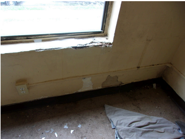
63. 260-268 Yamacraw Village - Unit 264 - 2-bed/ 1-bath TH - Plaster wall damage (Non-Critical Repair)
