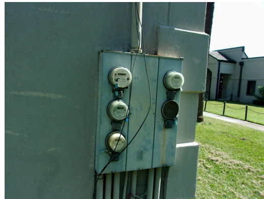
Typical electrical meter bank
