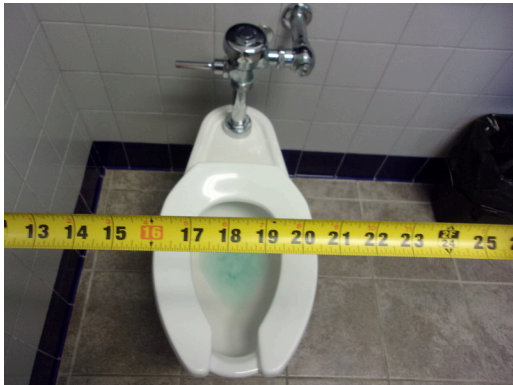
349 West Bryan Street - 2nd floor Doctor's office - Men's public restroom - Clear floor space at toilet
