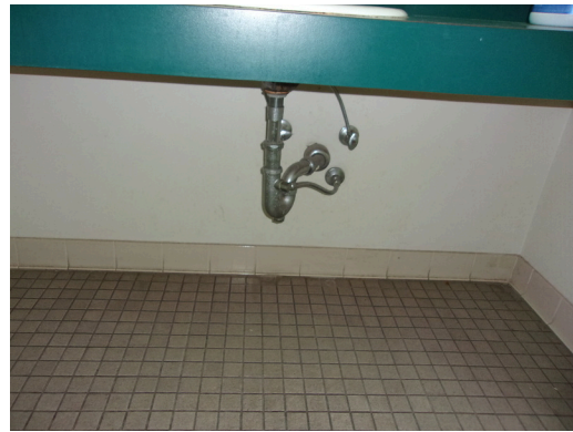
555 West Bay Street Office - Men's public restroom - No scald and abrasion protection at sink (Critical Repair)
