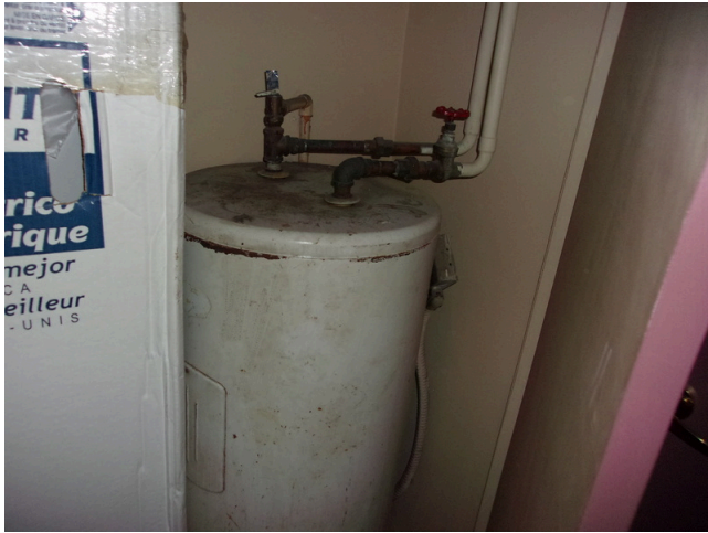
153. 349 West Bryan Street - Community center - Replace old 50-gallon water heater (Non-Critical Repair)
