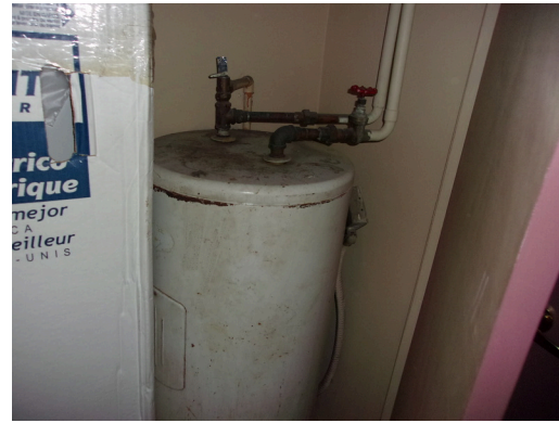
349 West Bryan Street - Community center - Replace old 50-gallon water heater (Non-Critical Repair)
