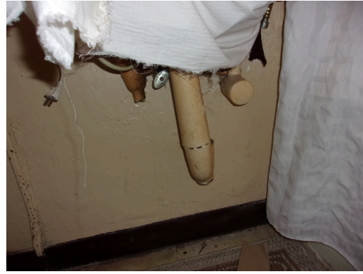
260-268 Yamacraw Village - Unit 261 - 1-bed/ 1-bath - HC unit - Partial scald and abrasion at sink
