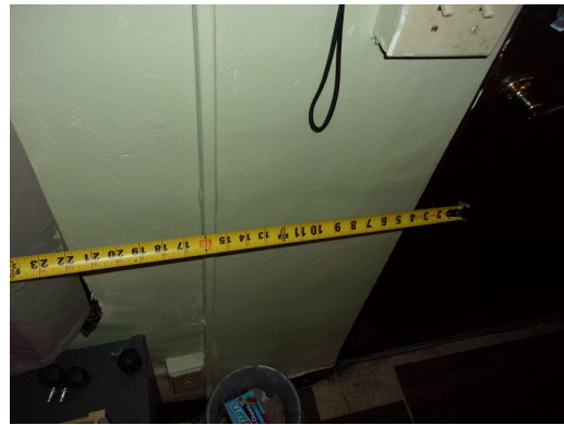
260-268 Yamacraw Village - Unit 261 - 1-bed/ 1-bath - HC unit - Adequate space at latch side of door
