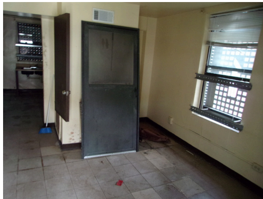
460-467 Yamacraw Village - Unit 461 - 1-bed/ 1-bath - HC unit/Down unit - Living room view, replace flooring (Non-Critical Repair)
