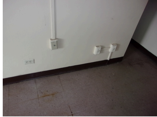
121-128 Yamacraw Village - Unit 126 - 2-bed/ 1-bath TH - Cable and electrical outlets
