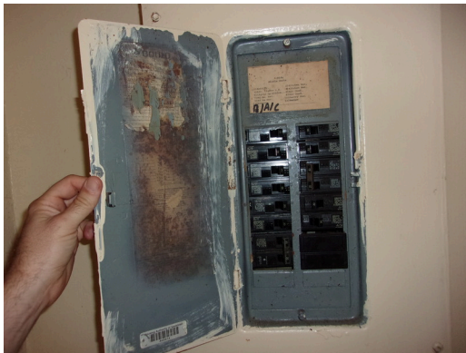
121-128 Yamacraw Village - Unit 126 - 2-bed/ 1-bath TH - Breaker panel
