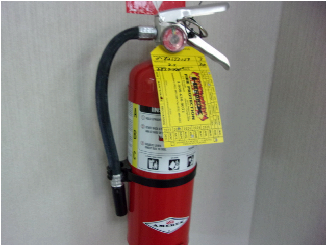
145. 555 West Bay Street Office - Fire extinguisher - Tag dated July 2023
