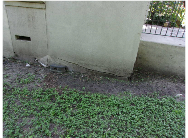
26. Evidence of foundation settling, damaged stucco siding (Non-Critical Repair)
