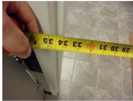
349 West Bryan Street - 2nd floor Doctor's office - Men's public restroom - 34 inch clear opening at HC stall door
