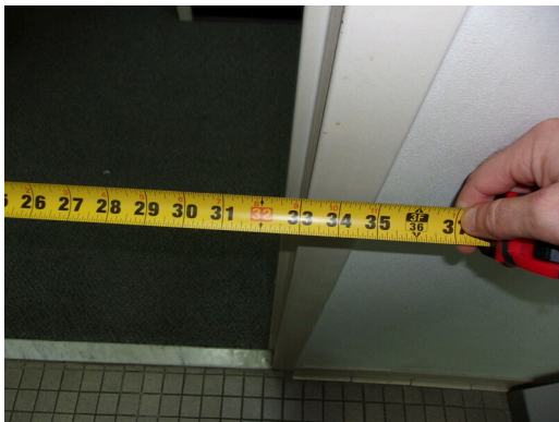
555 West Bay Street Office - Women's public restroom - 32 inch clear opening at door
