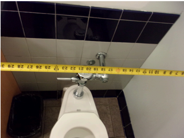
119. 349 West Bryan Street - 2nd floor Doctor's office - Men's public restroom - ADA signage
