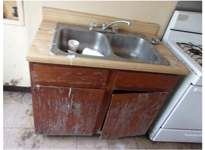
62. 260-268 Yamacraw Village - Unit 264 - 2-bed/ 1-bath TH - Replace cabinetry and fixtures (Non- Critical Repair)
