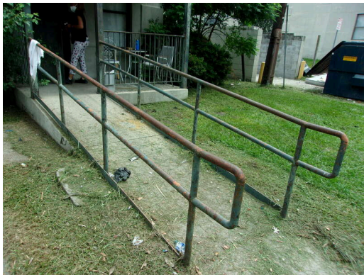
260-268 Yamacraw Village - Unit 261 - 1-bed/ 1-bath - HC unit - Replace metal/concrete ramp (Non-Critical Repair)
