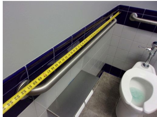
349 West Bryan Street - 2nd floor Doctor's office - Men's public restroom - Compliant side grab bar
