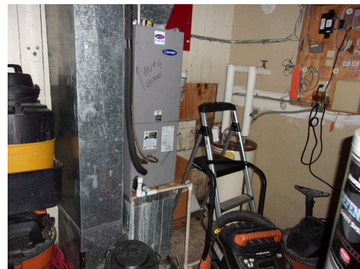
555 West Bay Street Office - Mechanical room with AHU and electric water heater
