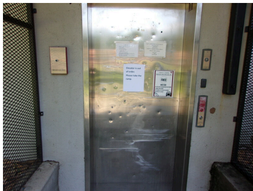
Hydraulic elevator at 349 West Bryan Street is not working and a certificate was not provided (Critical Repair)
