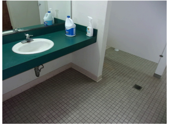
82. 555 West Bay Street Office - Men's public restroom - Replace common restroom accessories (Non-Critical Repair)
