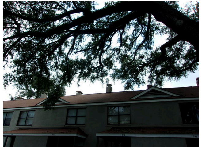
8. Typical trees touching apartment building roofs (Non-Critical Repair)
