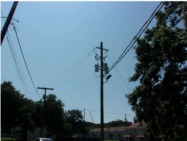
159. Pole mounted transformers
