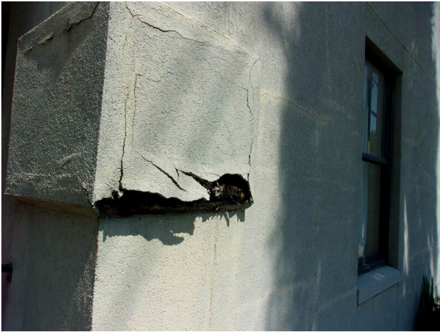
37. Damaged stucco siding (Non-Critical Repair)
