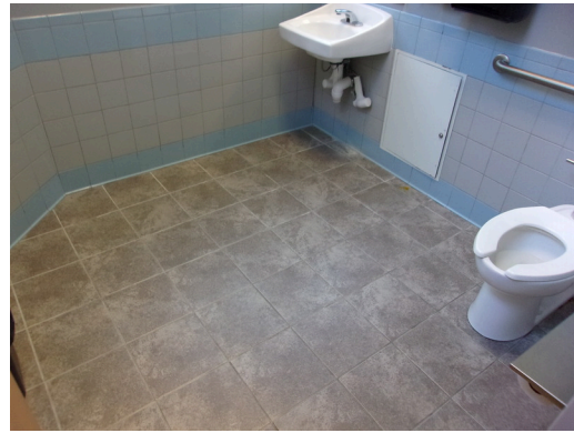
349 West Bryan Street - 2nd floor Doctor's office - Women's public restroom - HC stall view
