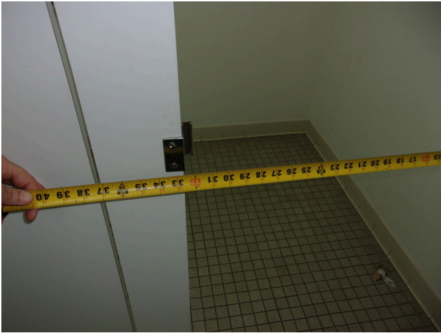
85. 555 West Bay Street Office - Men's public restroom - 32 inch clear opening at HC stall door
