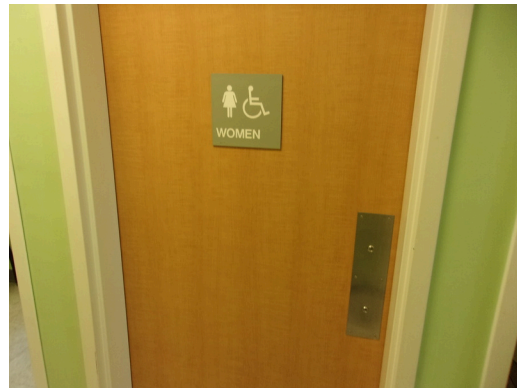
349 West Bryan Street - 2nd floor Doctor's office - Women's public restroom - ADA signage
