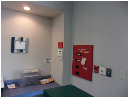
555 West Bay Street Office - Fire alarm - Provide annual report (Critical Repair)
