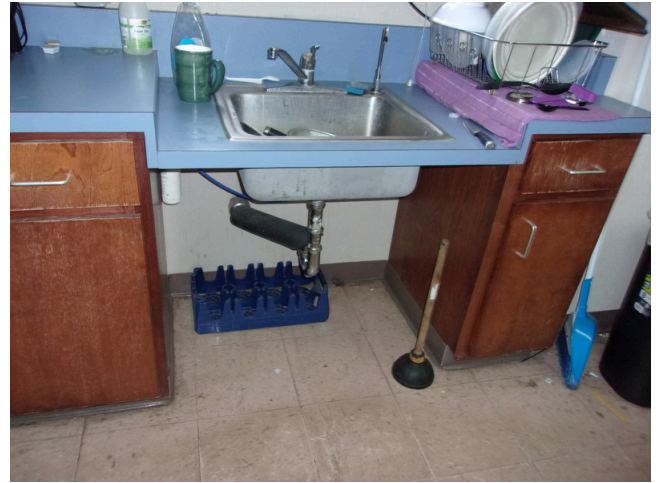
90. 555 West Bay Street Office - No scald and abrasion protection at kitchen sink (Critical Repair)
