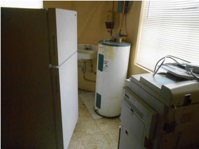
163. 349 West Bryan Street - Community center - Replace old 50-gallon water heater (Non-Critical Repair)
