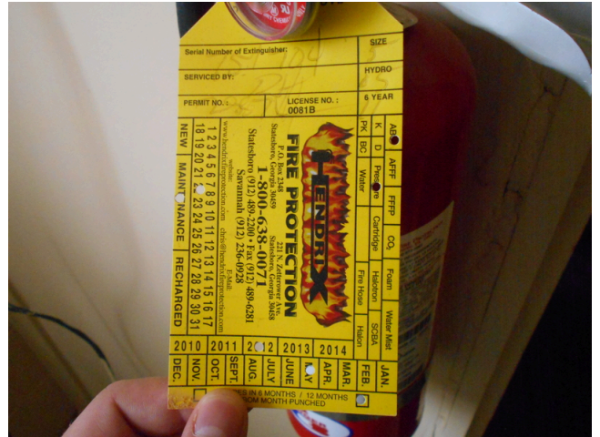
164. 349 West Bryan Street - Community center - Inspect fire extinguishers annually (Critical Repair)
