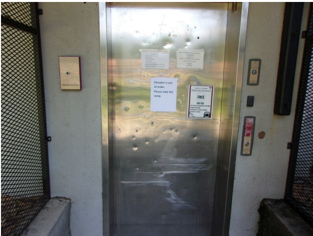
99. Hydraulic elevator at 349 West Bryan Street is not working and a certificate was not provided (Critical Repair)
