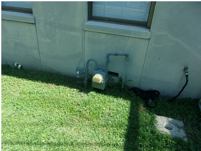
155. Typical gas meter
