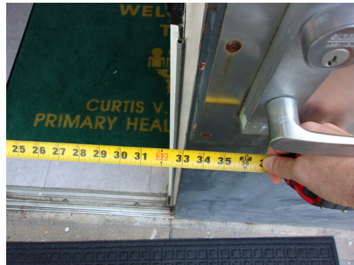
349 West Bryan Street - 2nd floor Doctor's office - 32 inch clear opening at door
