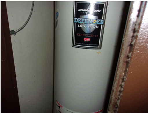
141-148 Yamacraw Village - Unit 142 - 3-bed/ 1-bath TH - Replace old water heater (Non-Critical Repair)
