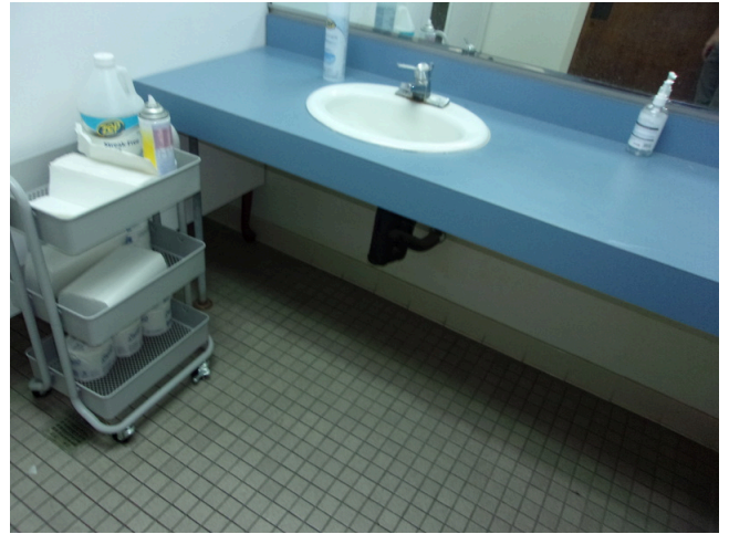
74. 555 West Bay Street Office - Women's public restroom - Levered sink with scald and abrasion protection, replace common restroom accessories (Non-Critical Repair)
