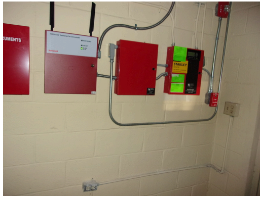
349 West Bryan Street - Community center - Fire alarm panel - Provide annual report (Critical Repair)
