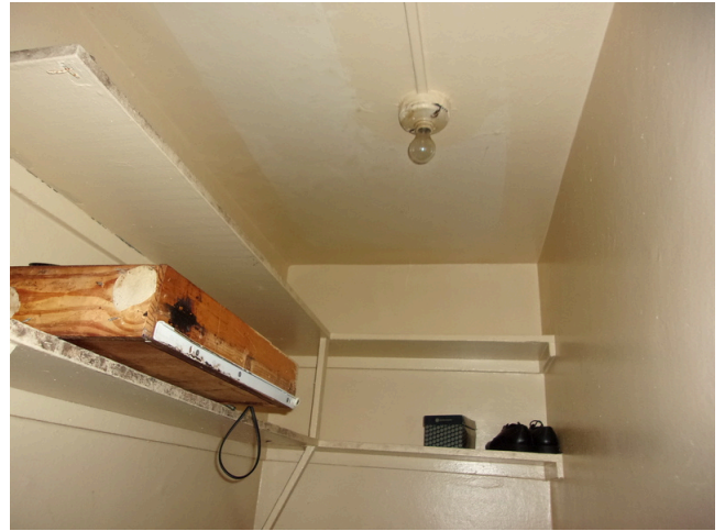
22. 141-148 Yamacraw Village - Unit 142 - 3-bed/ 1-bath TH - Replace old light fixtures (Non-Critical Repair)
