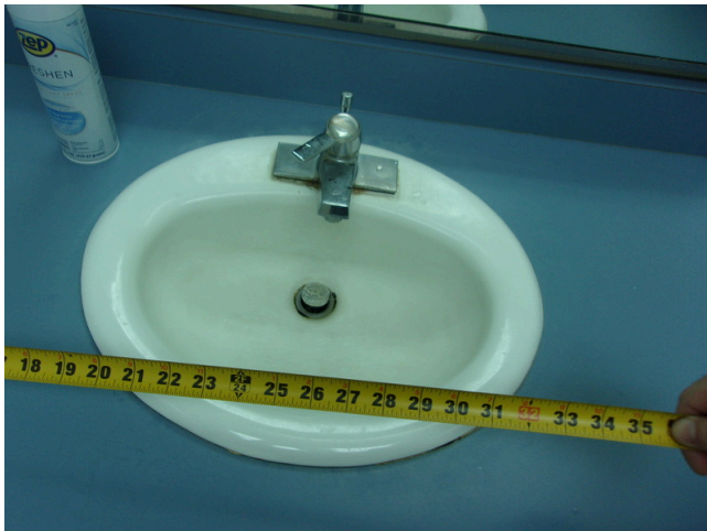
75. 555 West Bay Street Office - Women's public restroom - Clear floor space at sink
