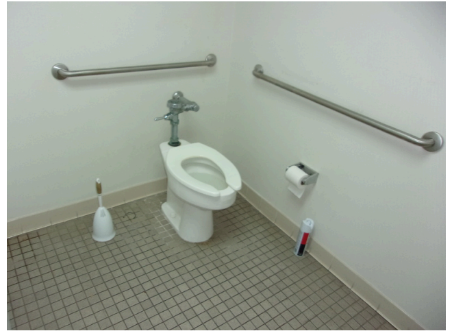
86. 555 West Bay Street Office - Men's public restroom - Toilet with compliant grab bars
