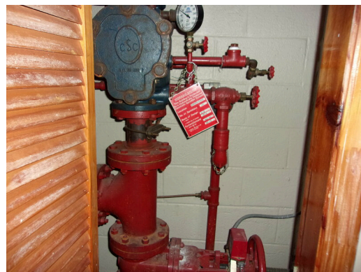
349 West Bryan Street - Community center - Fire riser - Provide annual sprinkler report (Critical Repair)
