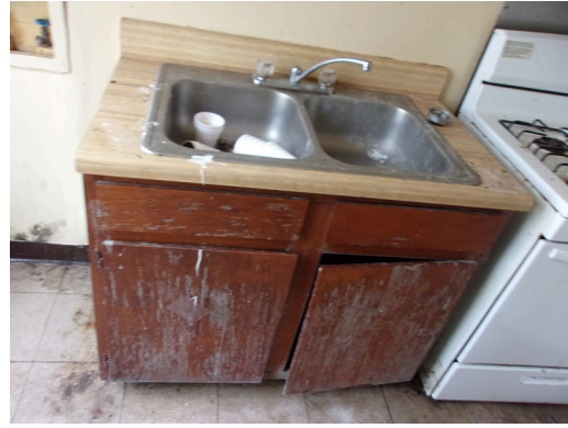
260-268 Yamacraw Village - Unit 264 - 2-bed/ 1-bath TH - Replace cabinetry and fixtures (Non-Critical Repair)
