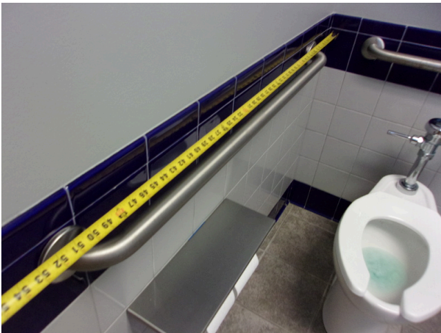
115. 349 West Bryan Street - 2nd floor Doctor's office - Men's public restroom - Compliant side grab bar
