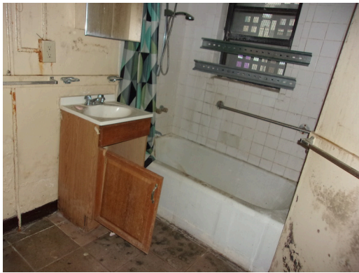
460-467 Yamacraw Village - Unit 461 - 1-bed/ 1-bath - HC unit/Down unit - Mold growth throughout, replace plumbing fixtures and vanity (Non-Critical Repair)
