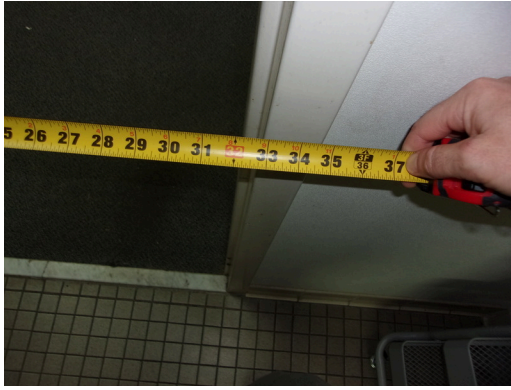
555 West Bay Street Office - Men's public restroom - 32 inch clear opening at door
