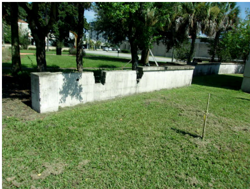
Replace damaged CMU retaining walls (Non-Critical Repair)
