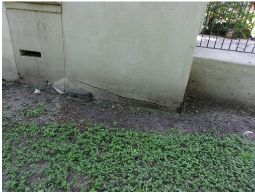
Evidence of foundation settling, damaged stucco siding (Non-Critical Repair)
