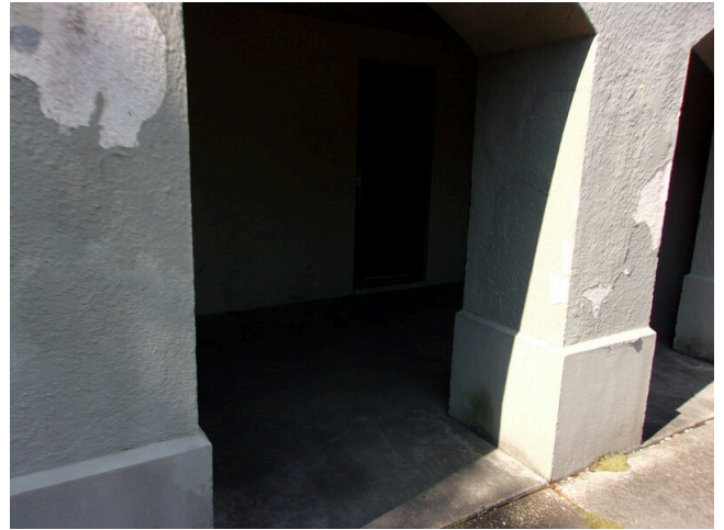
130. Repair and paint stucco siding at 349 West Bryant Street (Non-Critical Repair)
