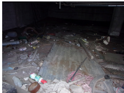
Crawlspace floor without vapor barrier
