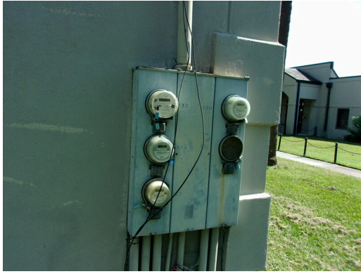
Typical electrical meter bank
