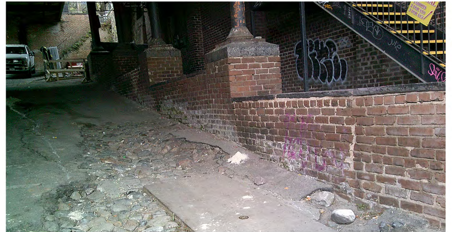
Poor condition of paving often collects small refuse and lends to a generally unkempt impression.
