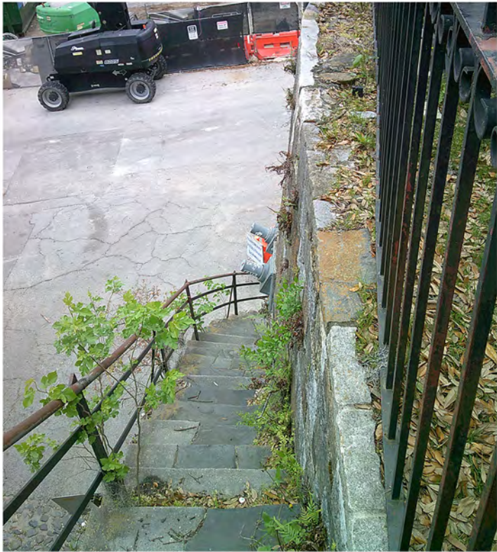
Closed stair from Emmett Park restricts pedestrian access between levels.
