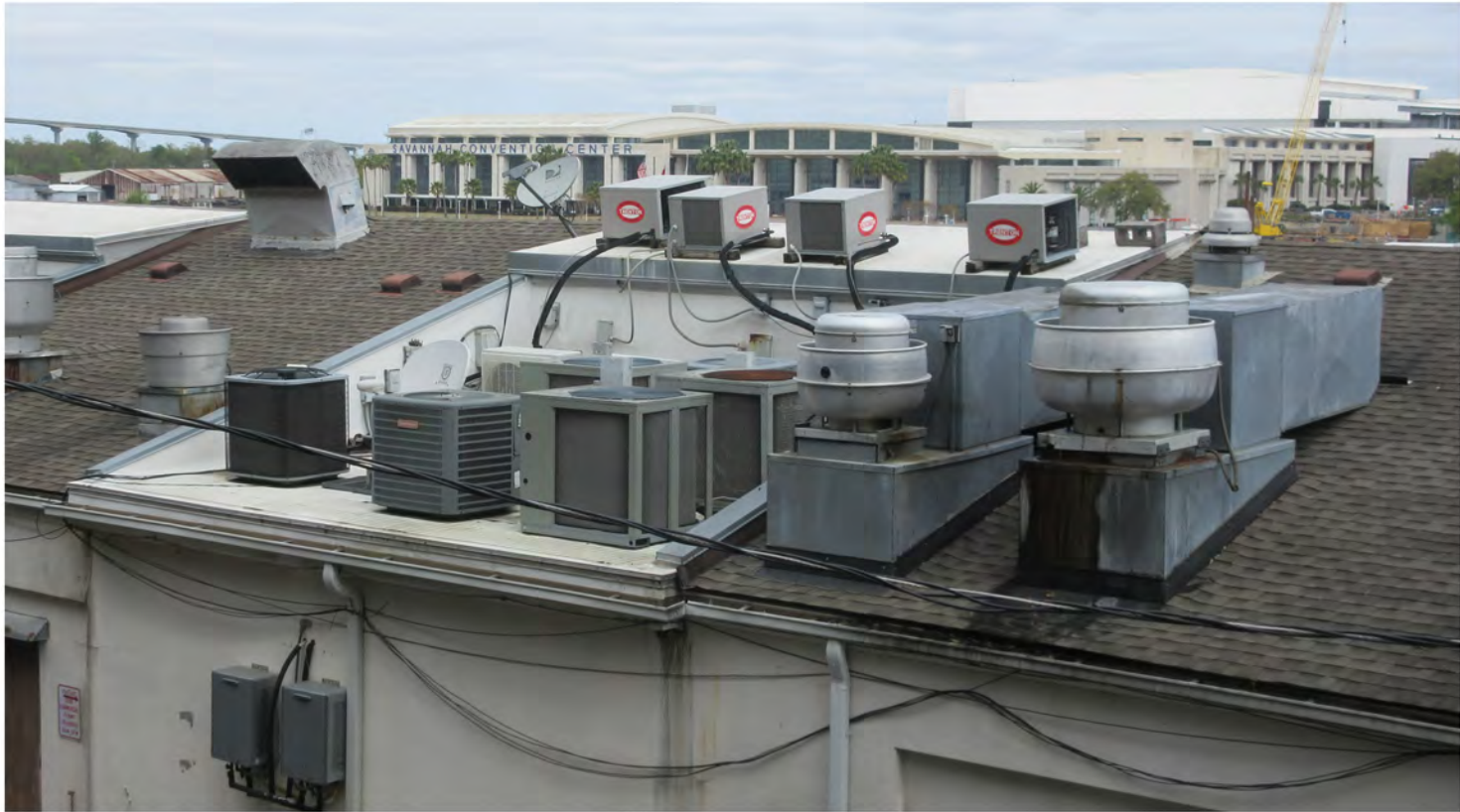
Rooftop utilities on the east end can be viewed from Emmet Park.
