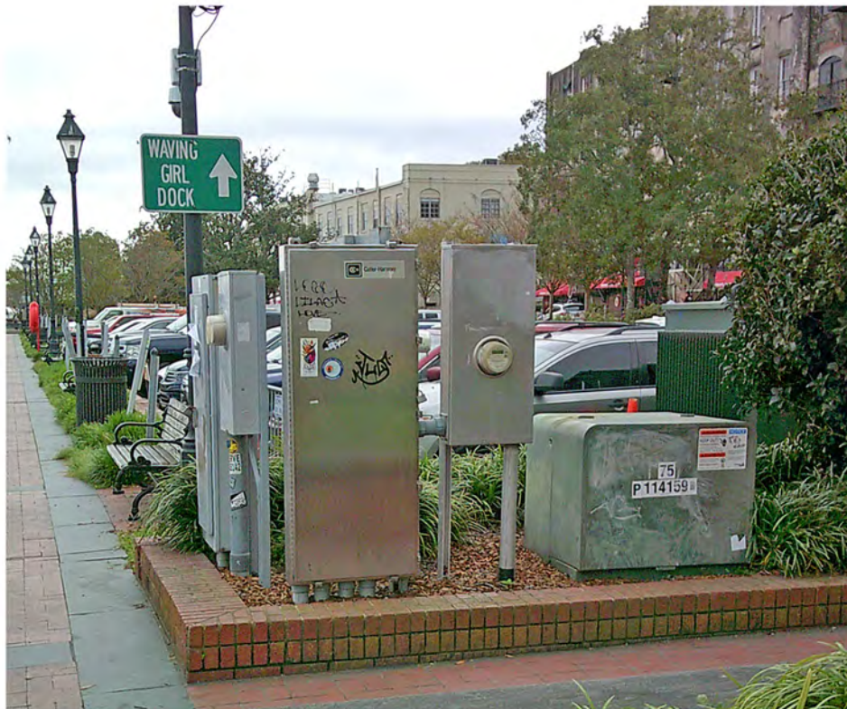
Landscaping is frequently interrupted by unsightly utility boxes.
