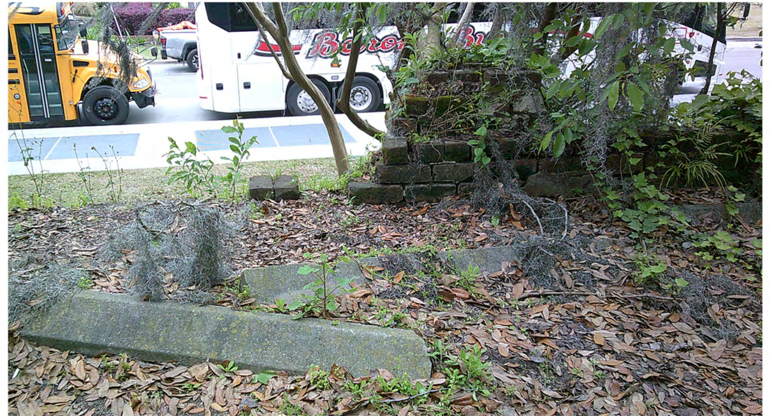
The retaining wall between Emmet Park and Morrell Park is disintegrating.
