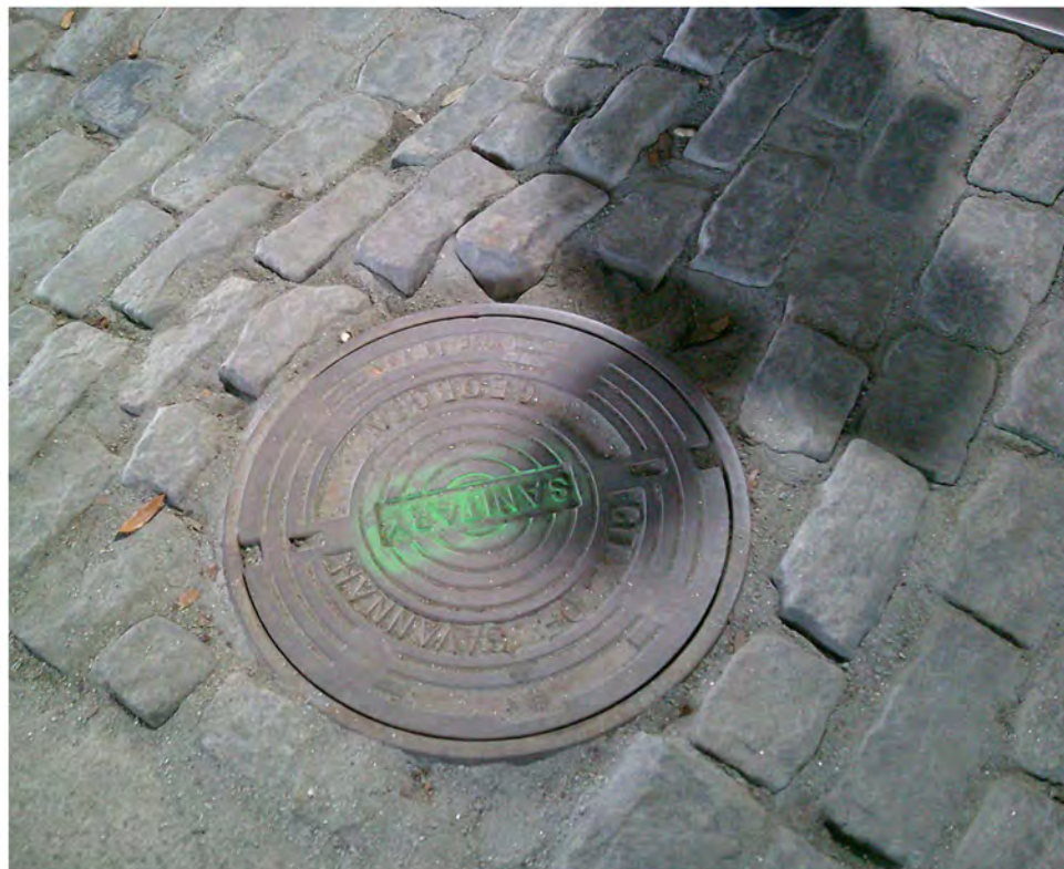
Uneven paving and abandoned signage can be hazardous to pedestrians.
