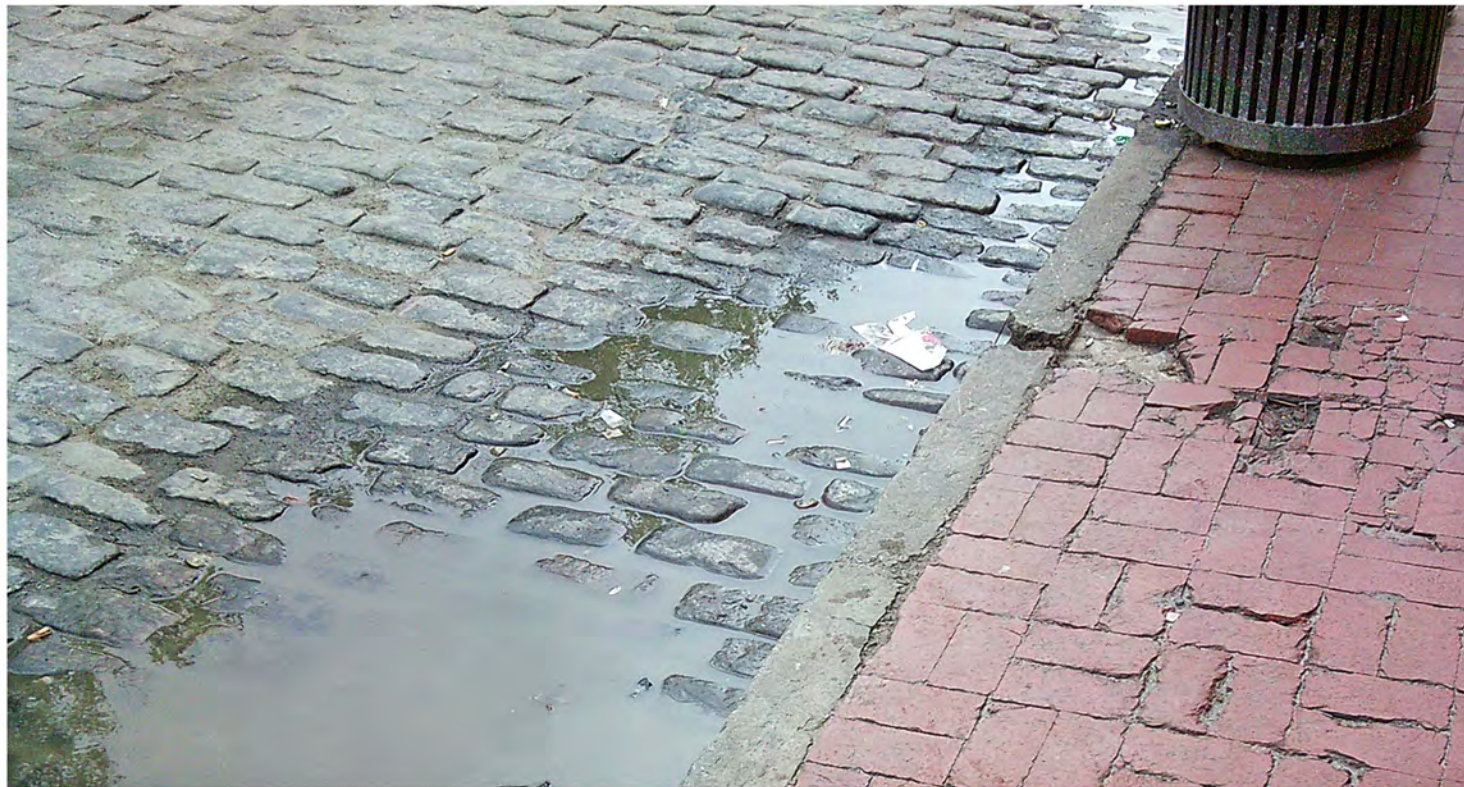
Standing water and uneven paving presents a problem, and frequently collect refuse.
