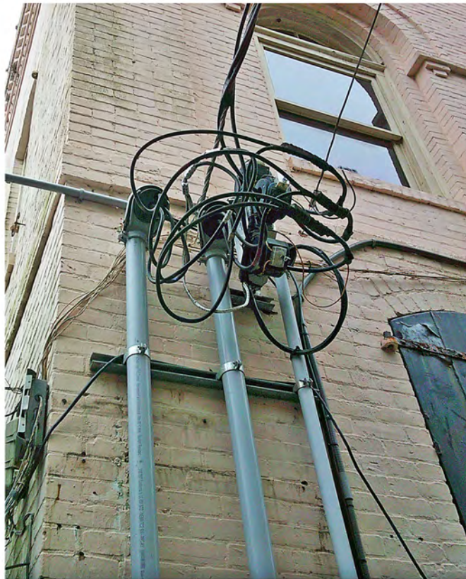
Cluttered electrical connections and exposed low-voltage and coaxial cables.
